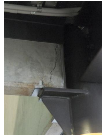
Figure 4: Shear failure at support of precast panel, shopping mall on Dilworth St and Clarence St, Christchurch [Photo by M. Bruneau].
