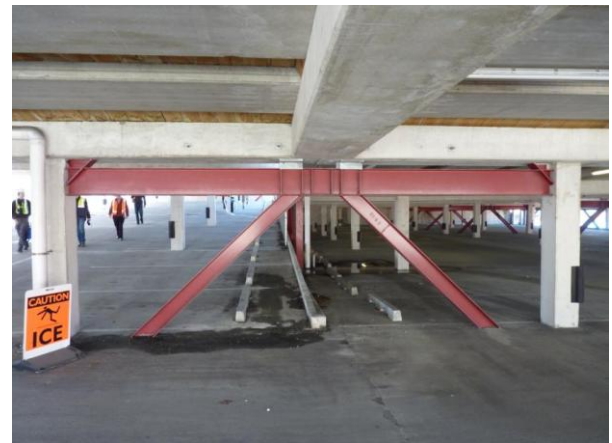
Figure 5: Typical bent in parking garage on St Asaph St and Antigua St, Christchurch (43°32'10"S-172°37'41"E) [Photo by M. Anagnostopoulou].
