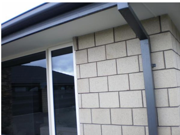
Figure 16: Light steel frame house from epicentral region [Photo Courtesy of Graham Rundle].
