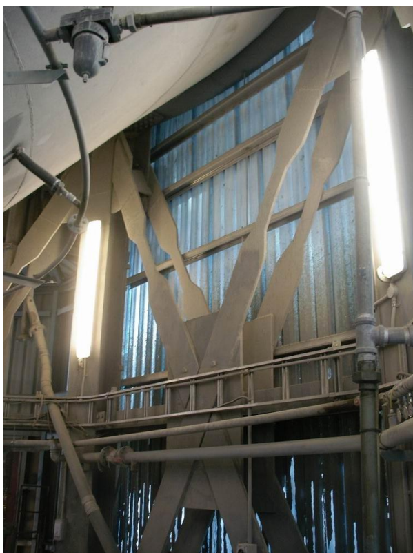
Figure 15: 2,000 tonne capacity cement Silo at Holcim Depot, Lyttleton, with deformed dogbone braces [Photo by Buchanan and Fletcher].
