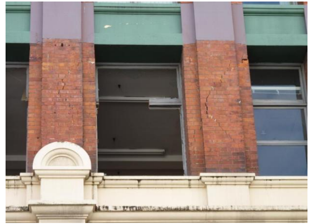
Figure 12: Damaged front piers of heritage building on Manchester St and Hereford St, Christchurch [Photo by M. Anagnostopoulou].
