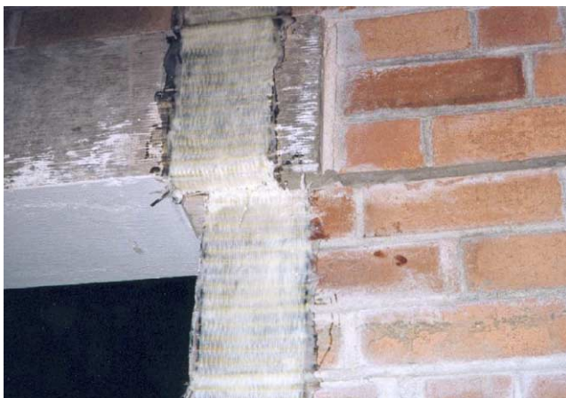
Fig. 13. Tyfo strip failed in shear.
