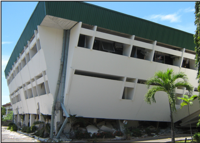
Figure 6. Soft story mechanism of a government office building in Padang
