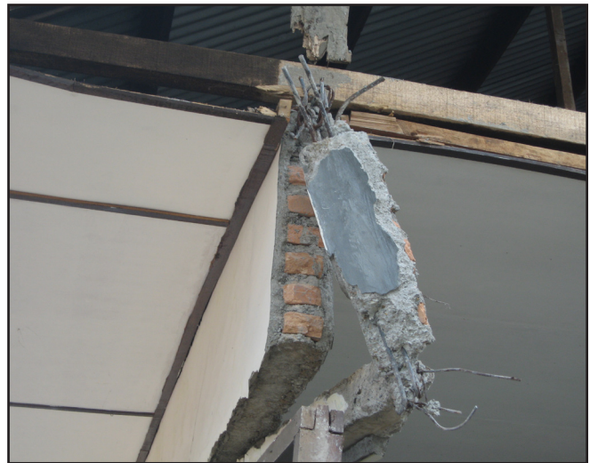
Figure 9. Failure of weak confining frame with poor detail (inadequate development/embedment length, sparse stirrups)
