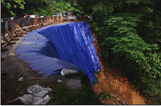
Figure 10. Slope stability failures of a road at Lubuk Selasih KM 18+00
