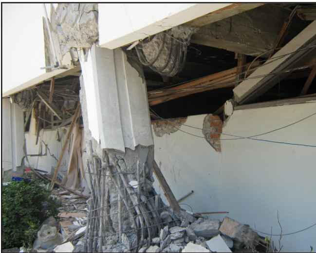
Figure 7. Poor detailing on RC structural members
