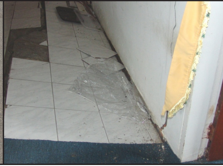
Figure 3. Foundation and ground deformations that caused damage to a building
