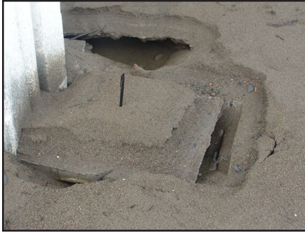
Figure 2. Example of liquefaction
