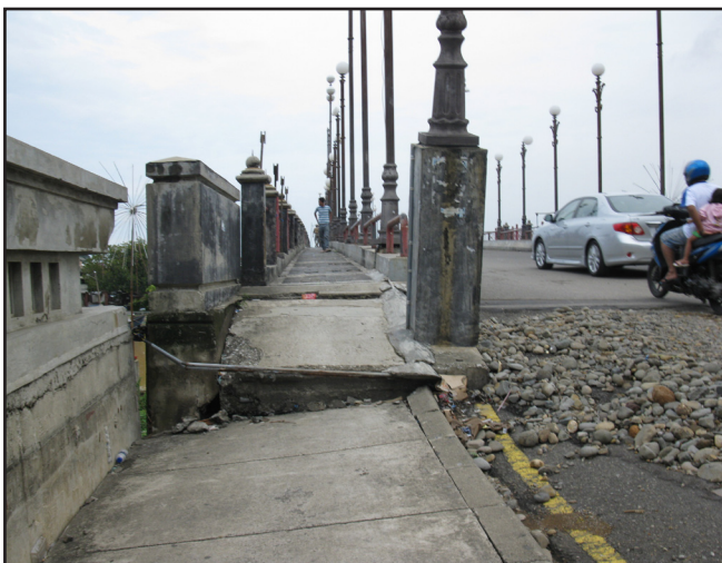
Figure 12. Damage to a bridge due to ground settlement within the fill of the approach and displacements of the abutment side walls
