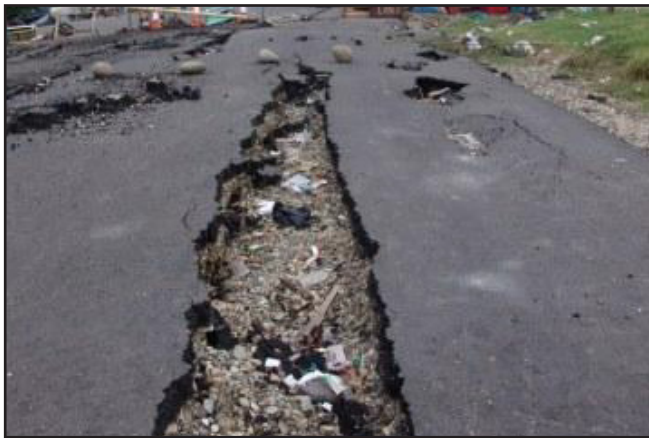
Figure 11. Damage to a road located along the shoreline in Padang due to lateral spread or slope stability of the road embankment
