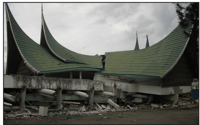
Figure 5. Total collapse mechanism of a government office building in Padang
