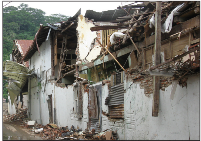
Figure 8. Damage to non-engineered structures in Padang
