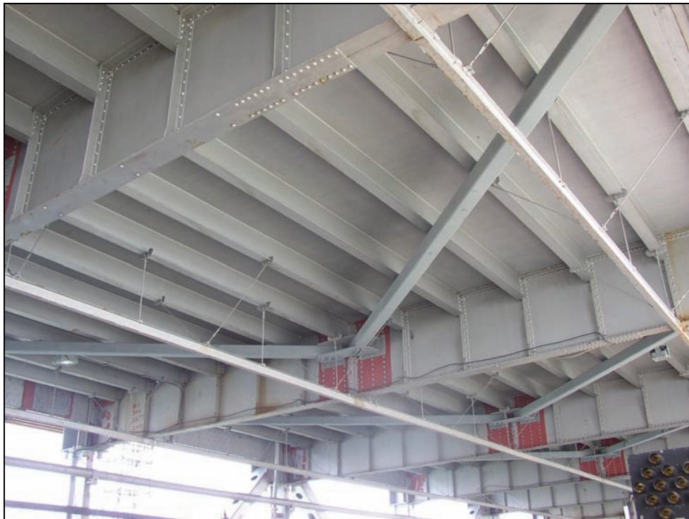
Figure 8-14. Typical Chevron Lateral Bracing Under the Deck of a Through Truss, Floor Beams and Stringers Support a Concrete Slab, the Three Rails Support a Maintenance Traveler
