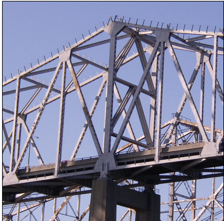
Figure 8-12. Cooper River Truss, Charleston, South Carolina, 1963 Main Tower Bearings and Vertical Lateral Bracing, Upper Chords Lateral Bracing System, and Safety Hand Railing on Upper Chords
