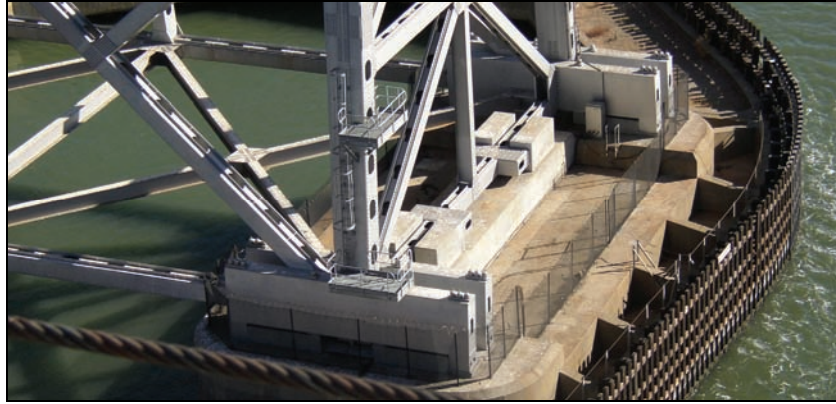
Figure 7-10. 1958 Carquinez Straits Truss Bridge showing Rocking Steel Box Beams that Provide Isolation and Damping of the Steel Braced Towers
