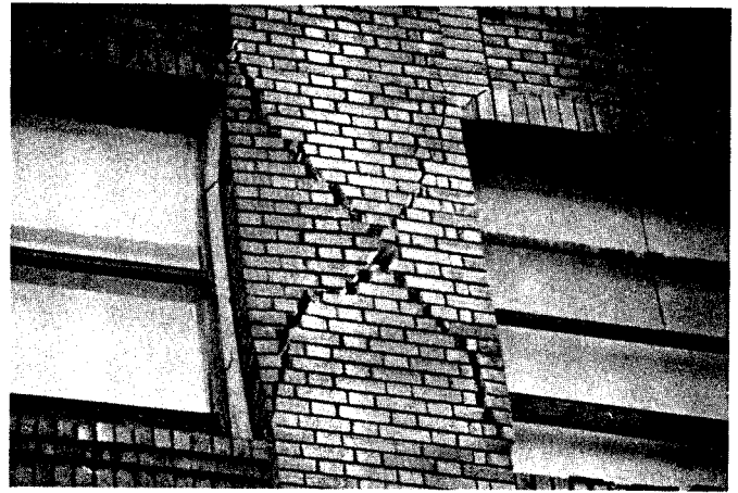
FIG. 13. Typical short column shear failure of masonry structure (Oakland).
