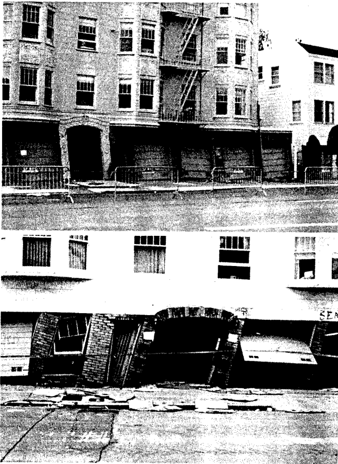
FIG. 12. Typical residential structures with "soft-story" problem (Marina district, San Francisco).
