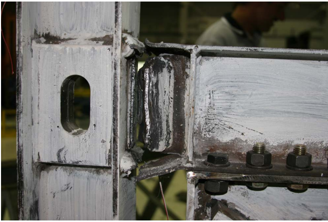
Fig. 14. Beam-to-column connection fracture
