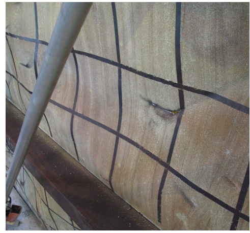
Photo 2 Steel plate buckling and cracks
