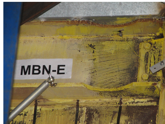
Photo 4 Middle Beam web yielding
