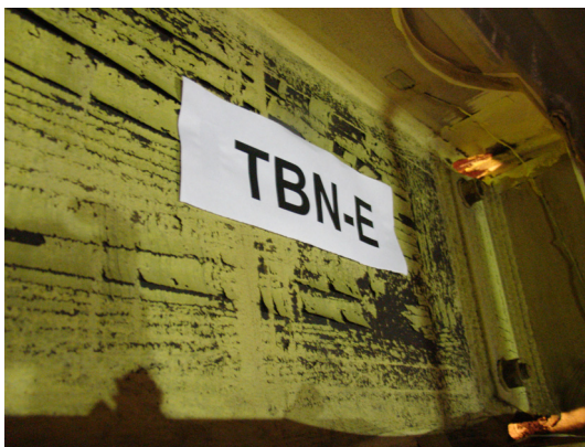
Photo 3 Top Beam web yielding
