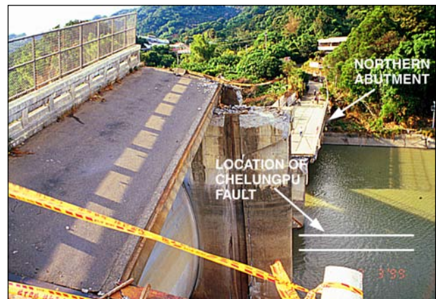
Figure 2a (top). View of northern end of Shih-kang Dam showing over 9 m of vertical offset at Chelungpu Fault and Figure 2b (bottom). View from uptrust side of Shih-kang Dam looking north.
