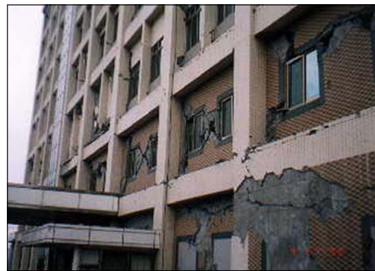
Figure 6. Damage to an exterior wall of the Shiu-Tuan Hospital in Nantou County.
