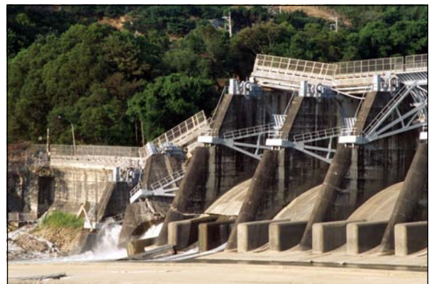
Surface faulting caused major damage to the Shih-kang Dam.
