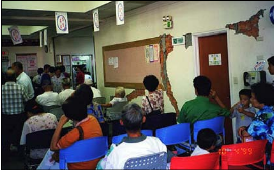
Figure 2. The first floor of the Christian Hospital remained open though the hospital suffered extensive interior damage.
