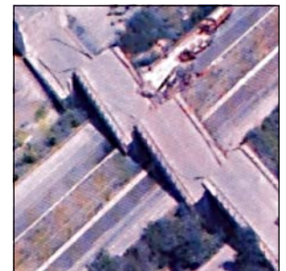
Figure 1. A collapsed overpass crossing the E80 Trans European Motorway near Adapazari. The fault rupture crossed beneath the bridge in the upper left portion of this photograph.
