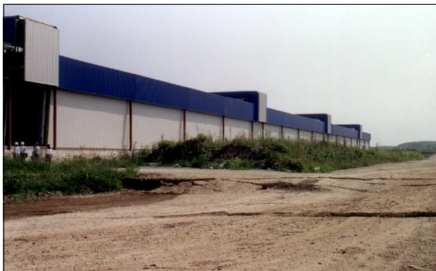
The fault rupture is visible next to this damaged manufacturing facility, under construction at the time of the earthquake.
