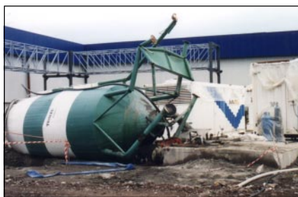
Figure 4. The anchor bolts ruptured and the unbraced support legs buckled, causing this water tank to tip.
