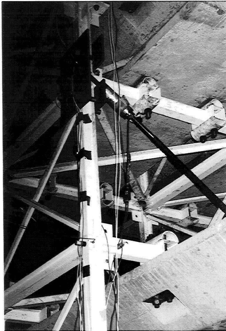
Figure 4-4 Photograph of the Third Floor-Tendon Connection: Load cells with a capacity of \pm 130 kN were installed in series with the tendon in order to record the supplementary system forces at this level. \Phi 25 mm-high strength threaded rods were used in the plate connections as shown.
