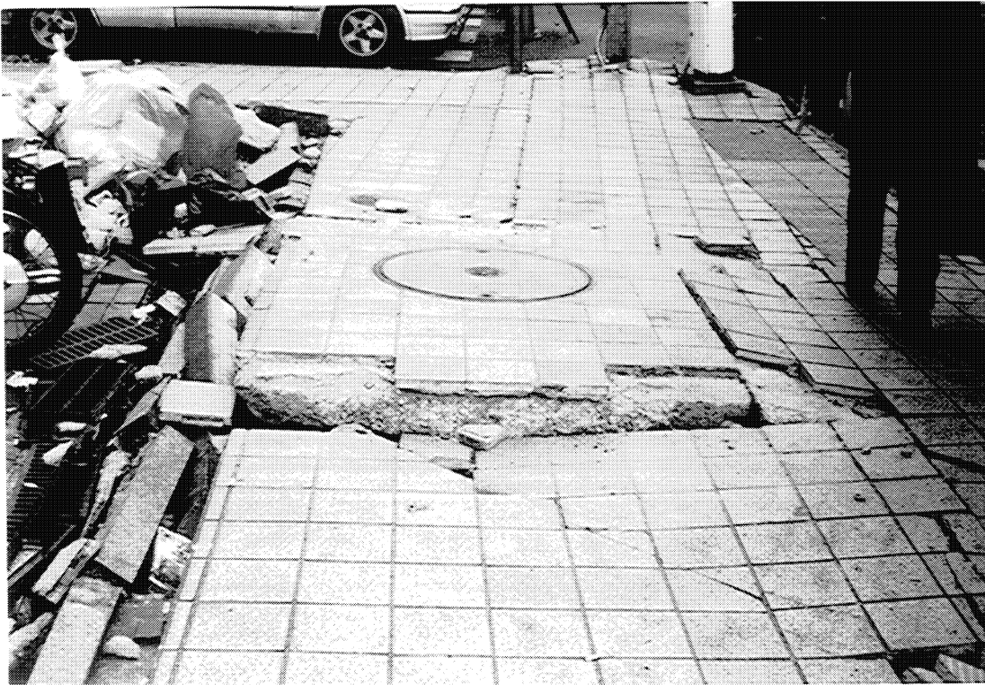
Figure 26 There was relative motion between this manhole and the surrounding soil. The relative motion could have been due to floating of the manhole or subsidence of the soil. Conduits connected to the manhole were damaged. (Kobe, Japan)
