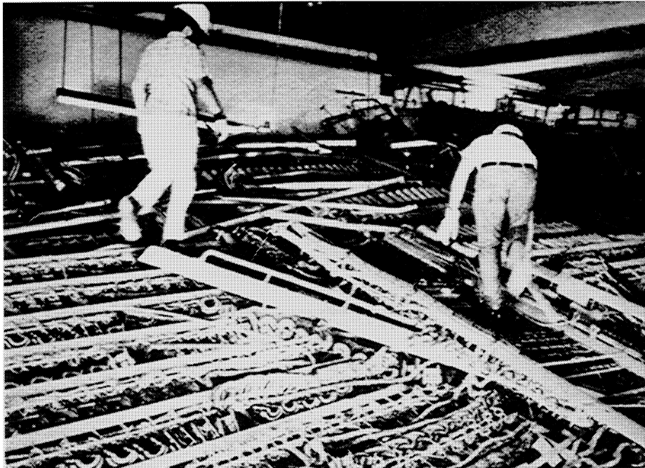
Figure 3 Switching equipment in a CO tipped over when overhead bracing and base anchors failed in a moderate earthquake. The equipment was a total loss and it took several months to replace and install new equipment. It took four days to install temporary lines to provide limited service until regular service could be restored.
