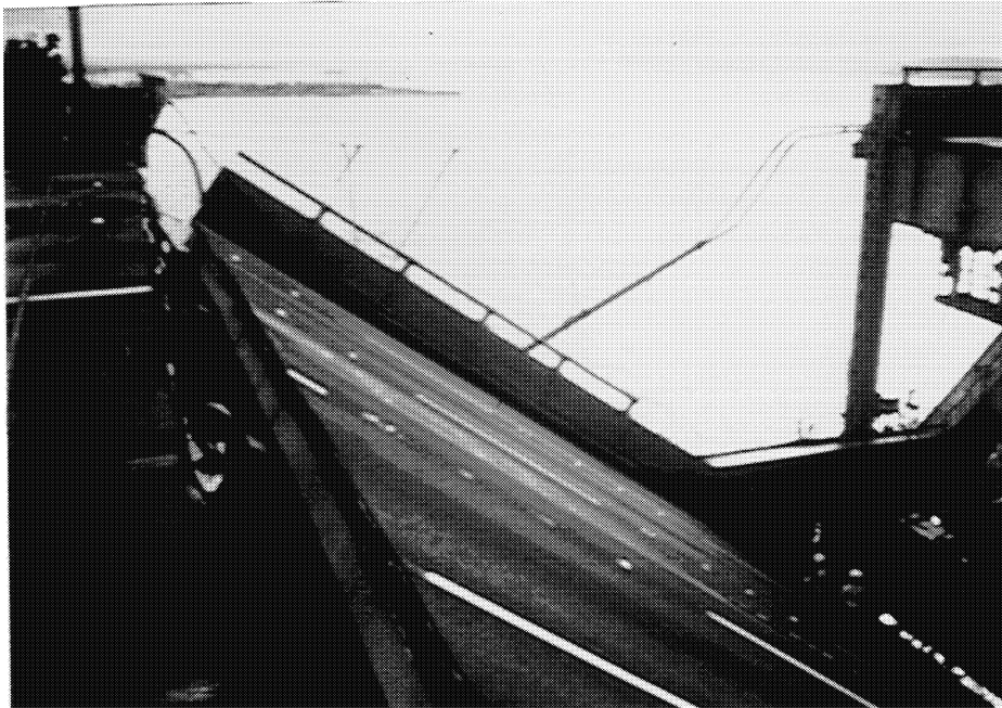
Figure 27 A section of the upper deck of the Bay Bridge between Oakland and San Francisco failed. A conduit that carried about 90 optical fibers was connected to the upper deck. The conduit broke away from the upper deck when it fell, and experienced significant deformation. Most of the optical fibers within the conduit were undamaged.
