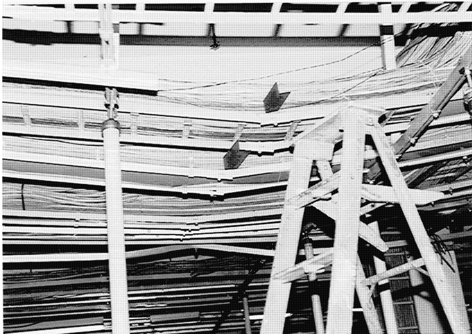
Figure 8 The buckling of the framing system at a splice demonstrated the lack of capacity of the friction clip splice.
