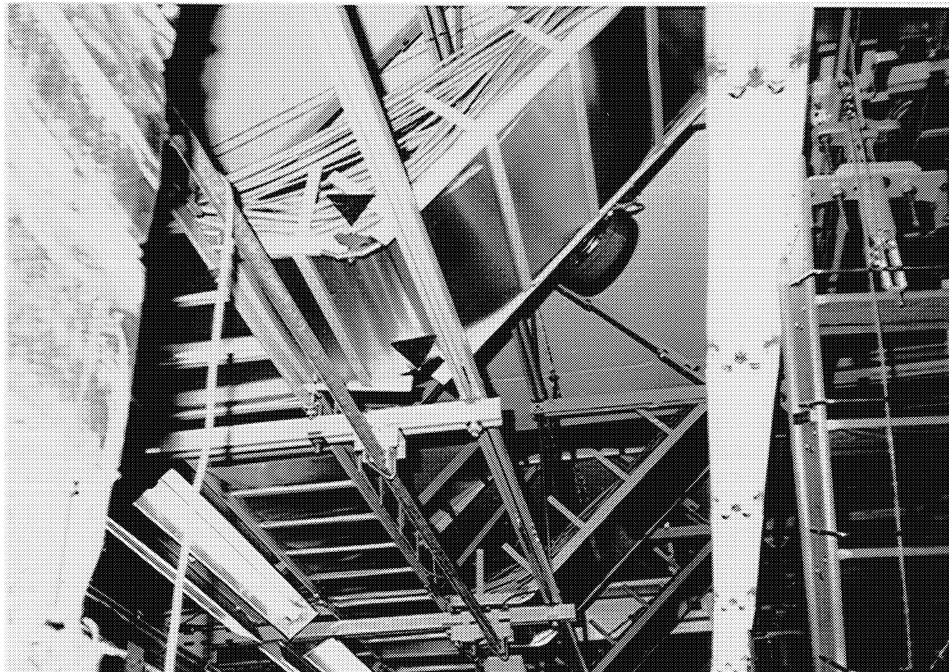
Figure 2 Friction clips used to splice cable racks together have pulled out in earthquakes. A positive structural connection is the preferred method of splicing.
