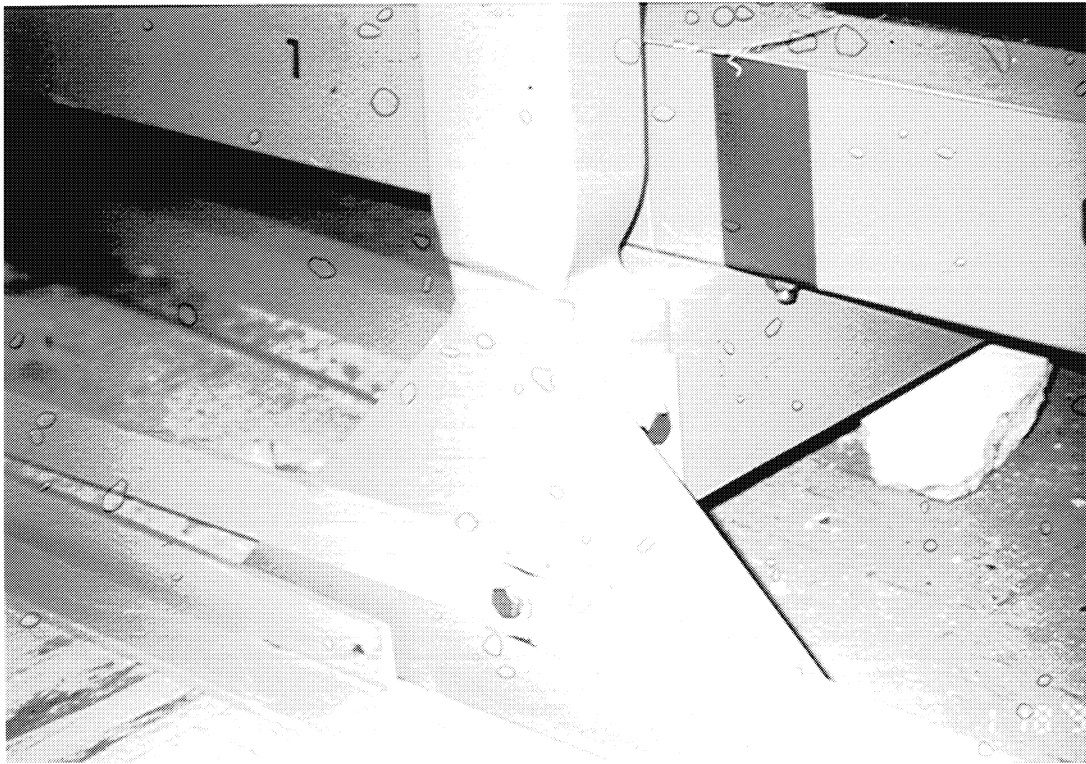
Figure 13 One of the standard battery racks failed because it was fabricated from thin sheet metal and had inadequate gussets.
