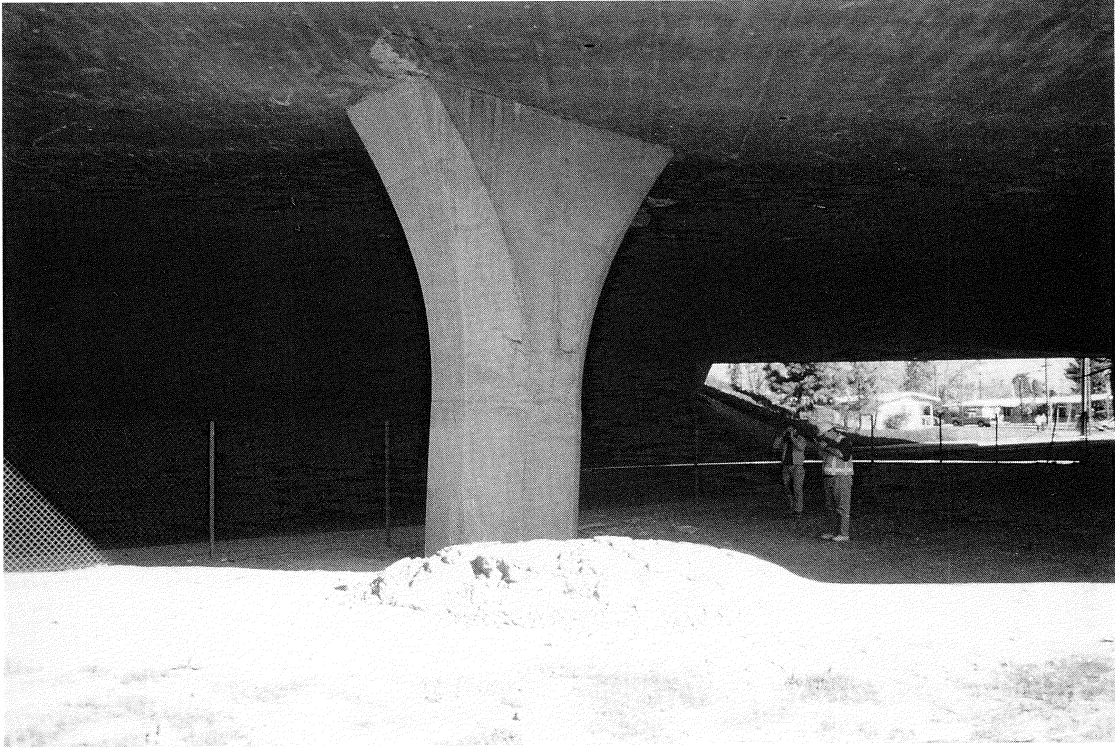
FIGURE 7-9 Mission-Gothic Undercrossing - Soil Upheaval Above Footing of Right Hand Column in Bent 2 of Eastbound Bridge
