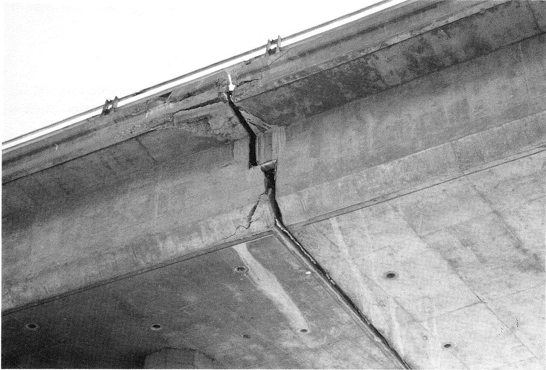
FIGURE 12-1 SR14/I-5 South Connector - Pounding and Damage to Hinge Seat in Span 6
