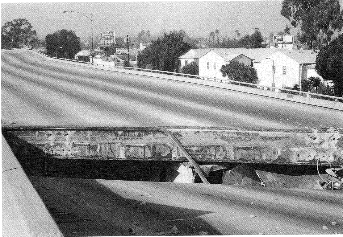
FIGURE 10-6 La Cienega-Venice Undercrossing - Unseated Hinge Near Bent 6
