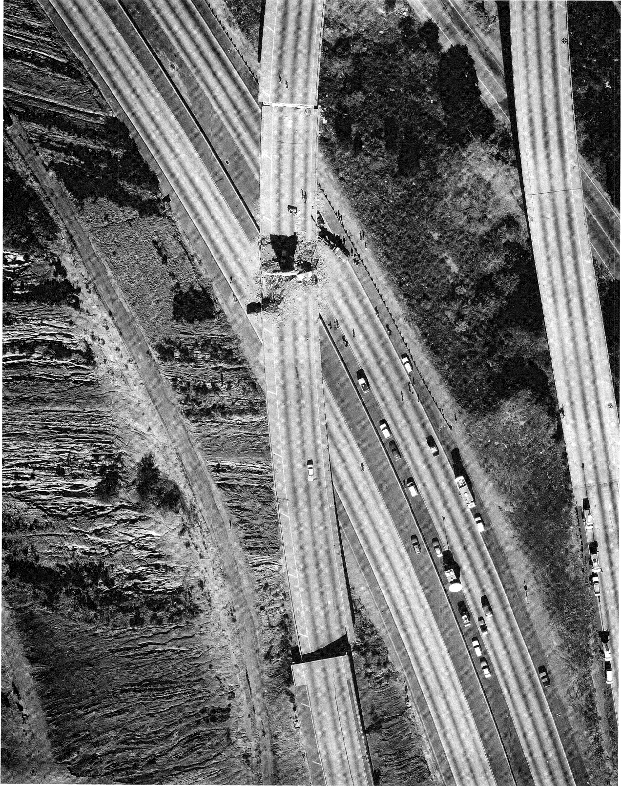
FIGURE 4-7 SR14/I-5 Separation and Overhead (Southbound) - Aerial View of Collapse
