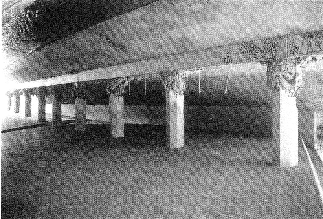
FIGURE 6-5 Bull Creek Canyon Channel Bridge - Hinges in All Columns of Bent 3 Immediately Above the Channel Training Wall
