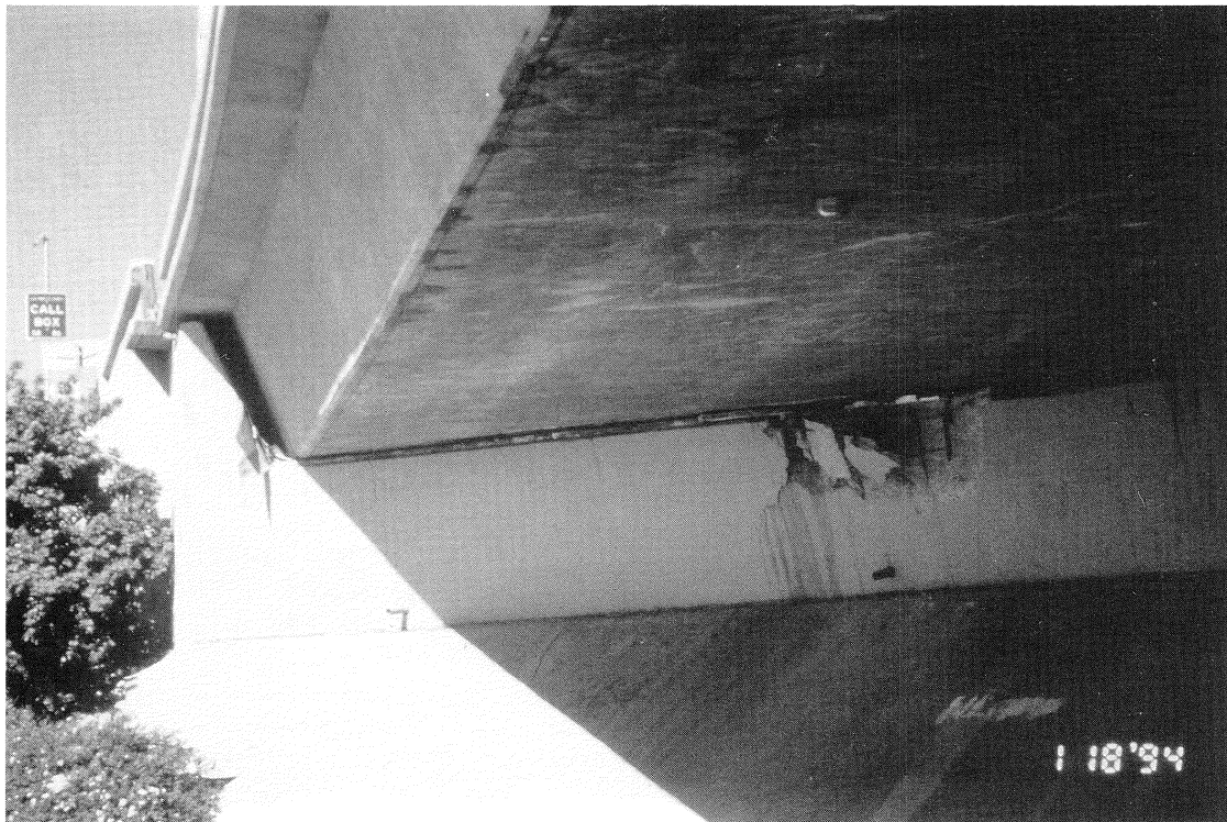
FIGURE 7-8 Mission-Gothic Undercrossing - Shear Key Damage at West Abutment of Eastbound Bridge
