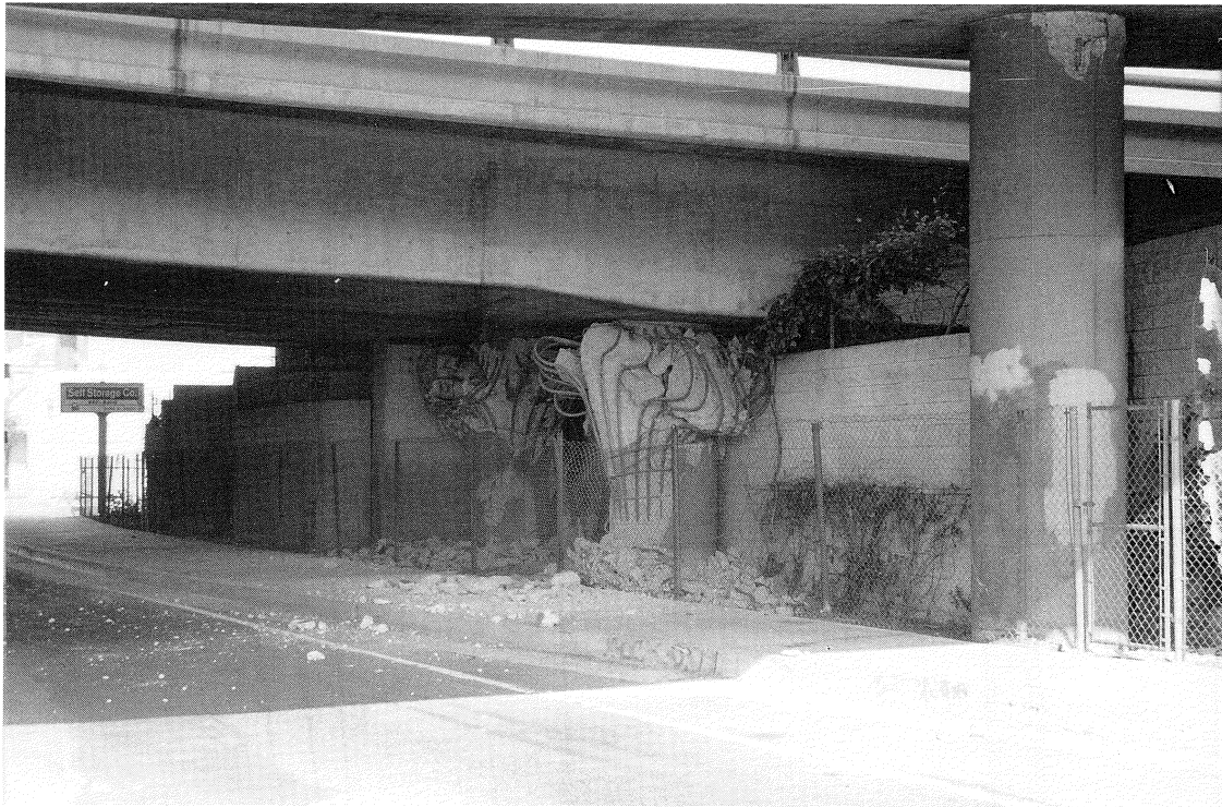
FIGURE 10-2 La Cienega-Venice Undercrossing - Column Failure in Bent 3
