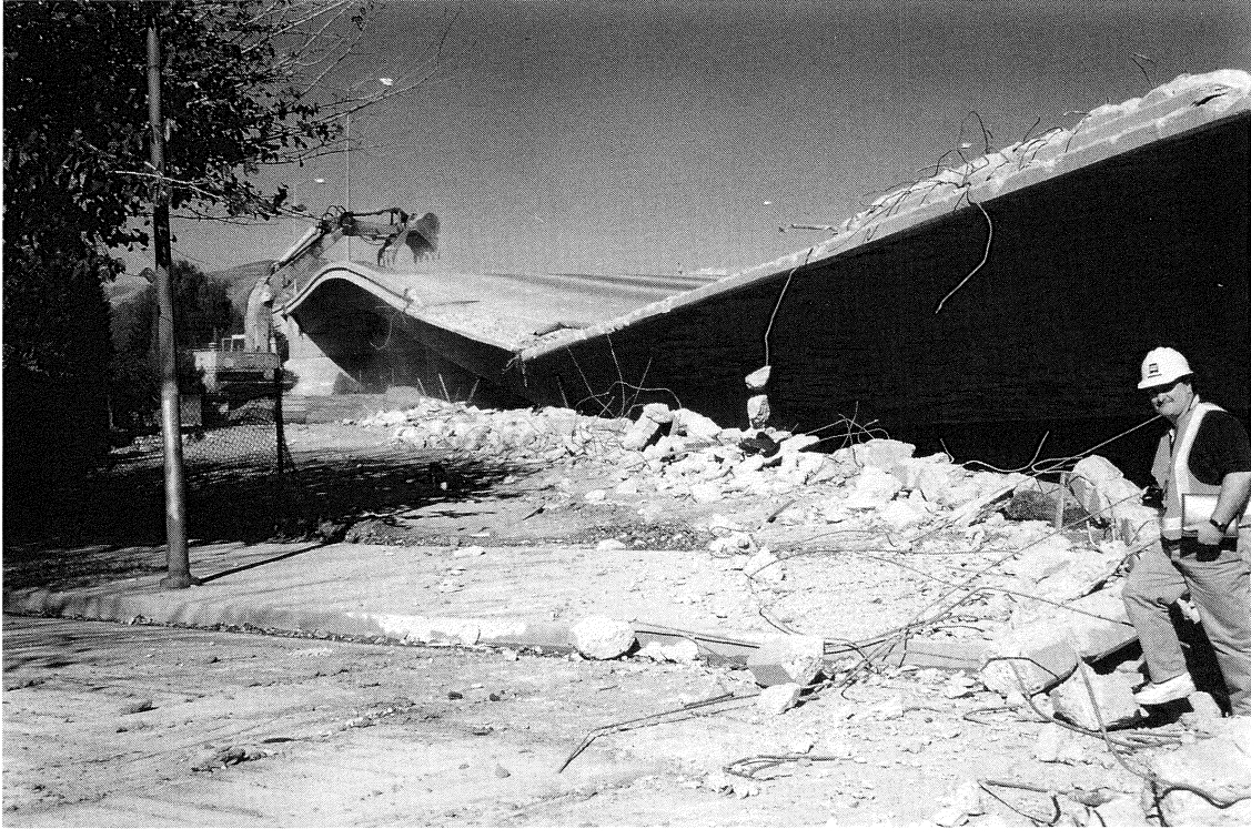
FIGURE 7-3 Mission-Gothic Undercrossing - Side View of Partially Collapsed Eastbound Bridge
