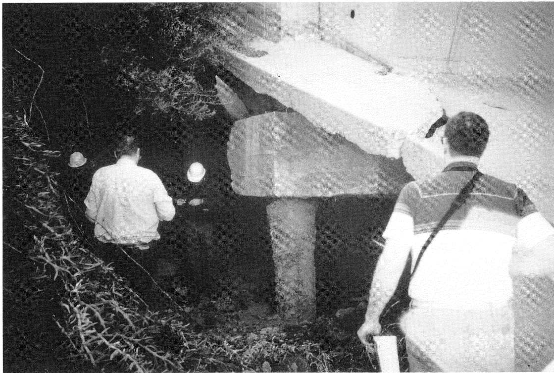
FIGURE 8-3 Balboa Boulevard Overcrossing - Soil Erosion at South Abutment Due to Ruptured Water Lines
