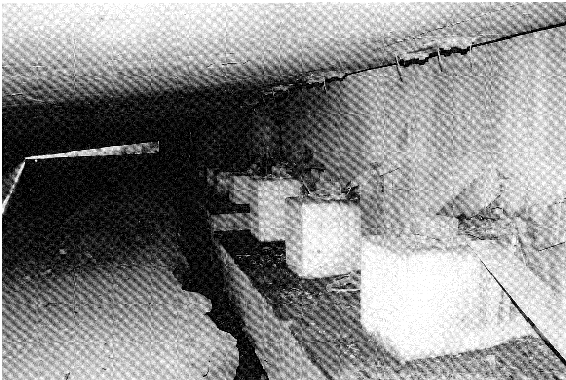
FIGURE 9-4 Fairfax-Washington Undercrossing - Uplift from Seat at Abutment 1
