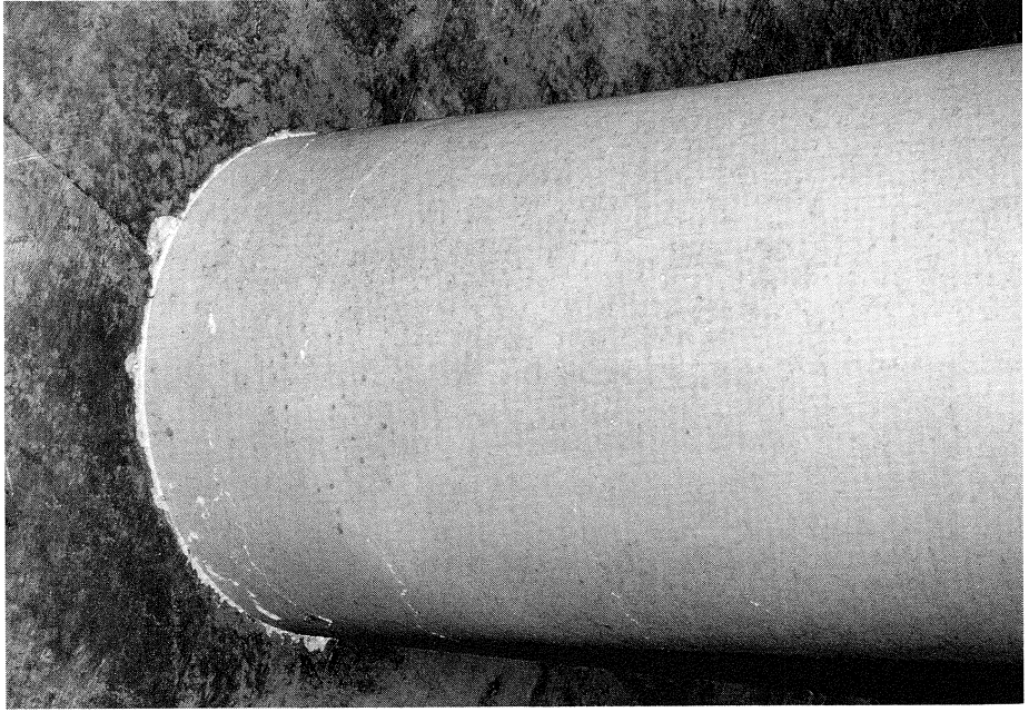
FIGURE 9-9 Fairfax-Washington Undercrossing - Minor Column Damage in Bent 5
