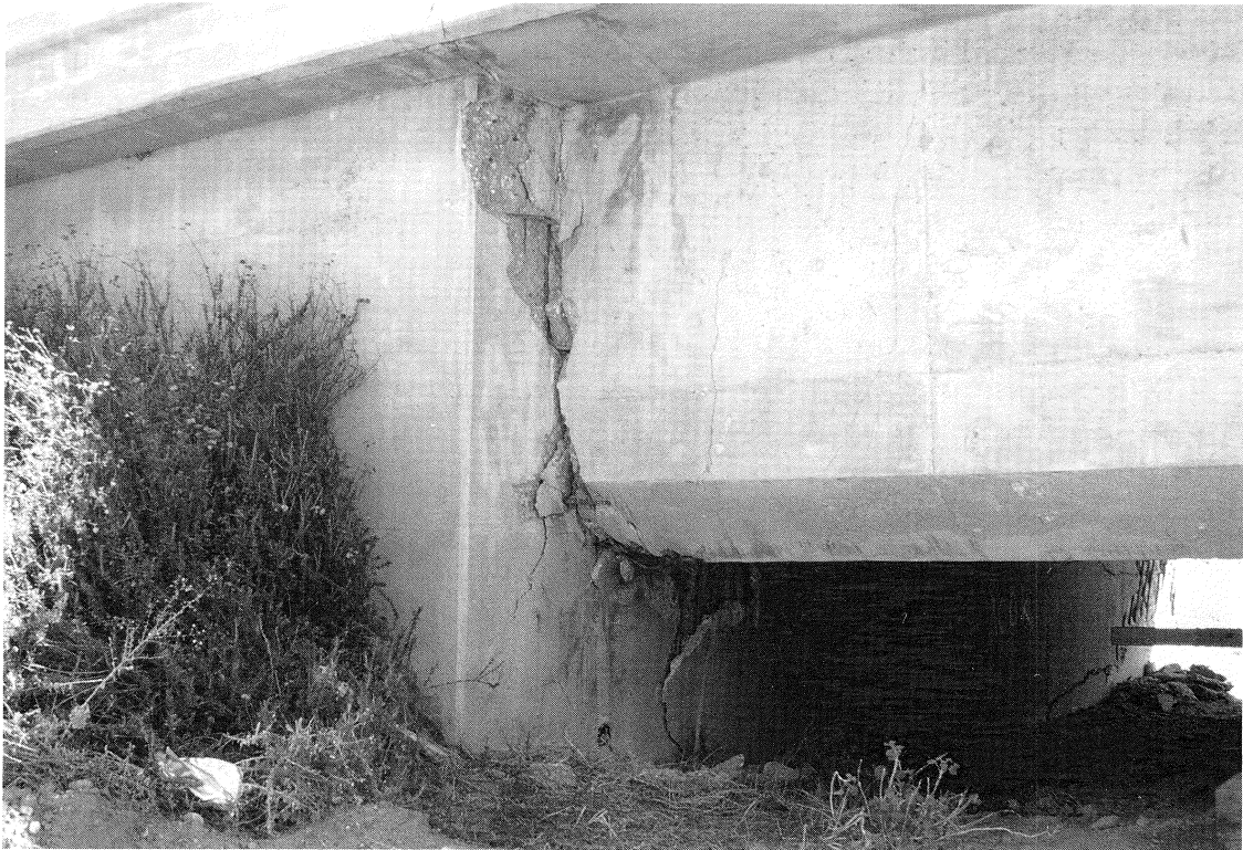
FIGURE 12-2 SR14/I-5 South Connector - Damage to Abutment 10
