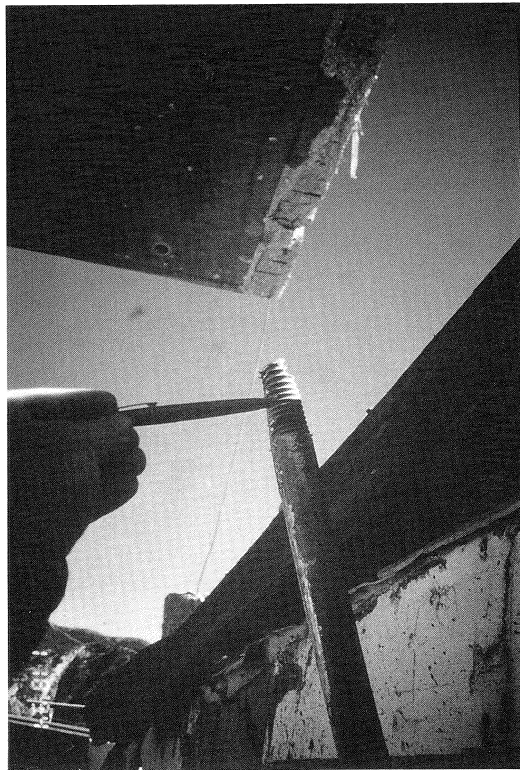
FIGURE 4-9 SR14/I-5 Separation and Overhead (Southbound) - Equalizing Bolt at Hinge in Span 3
