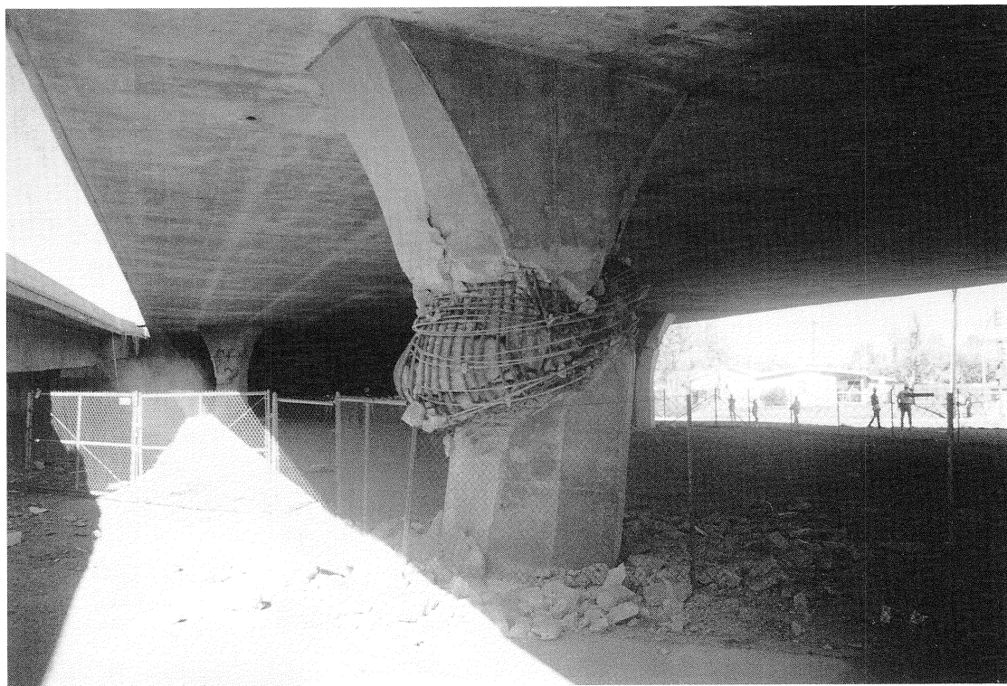
FIGURE 7-6 Mission-Gothic Undercrossing - Hinge Formation Below Flare in Column of Westbound Bridge (Face View)
