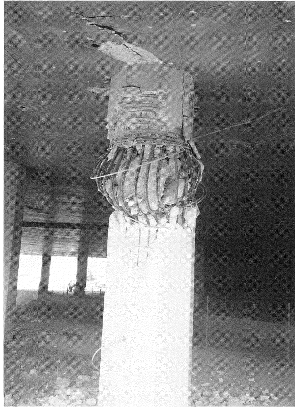
FIGURE 6-4 Bull Creek Canyon Channel Bridge - Hinge Formation Below Well Confined Section in Column of Bent 2 (Eastbound Bridge)
