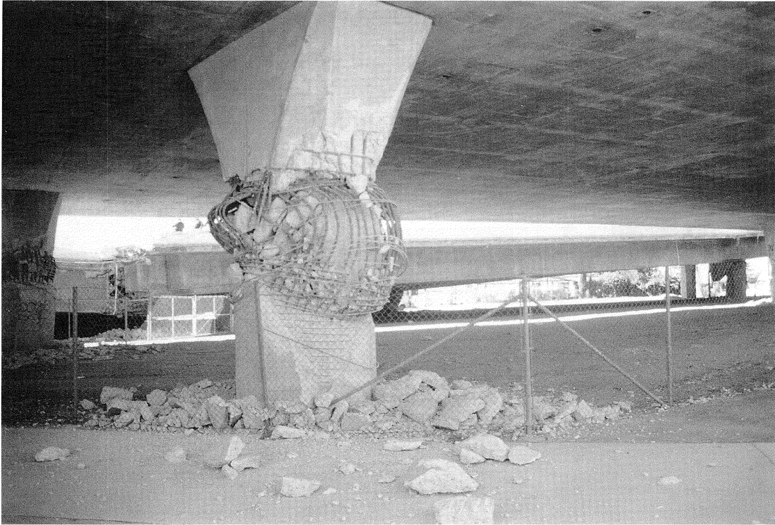
FIGURE 7-7 Mission-Gothic Undercrossing - Hinge Formation Below Flare in Column of Eastbound Bridge (Side View)
