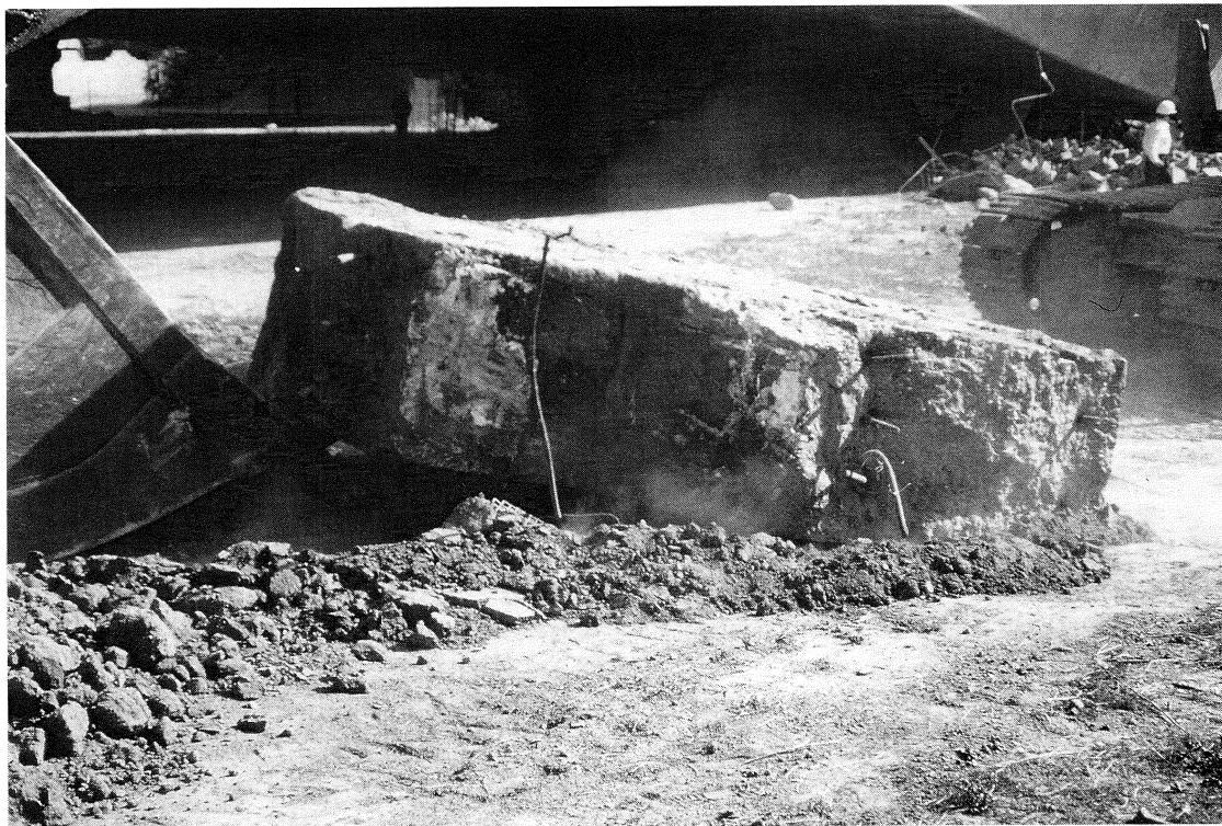
FIGURE 7-10 Mission-Gothic Undercrossing - Excavated Collar from Footing of Right Hand Column in Bent 2 of Eastbound Bridge
