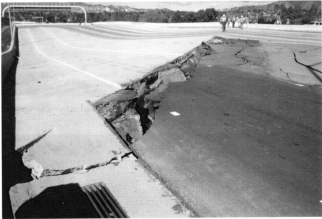
FIGURE 12-4 Bull Creek Canyon Channel Bridge - Slumping of Abutment Fills under Roadway Shoulders
