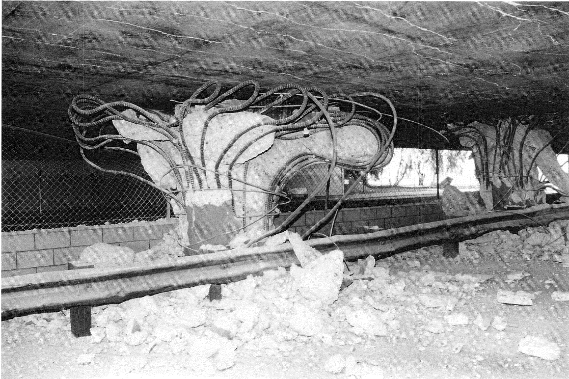
FIGURE 9-7 Fairfax-Washington Undercrossing - Total Column Failure in Bent 3
