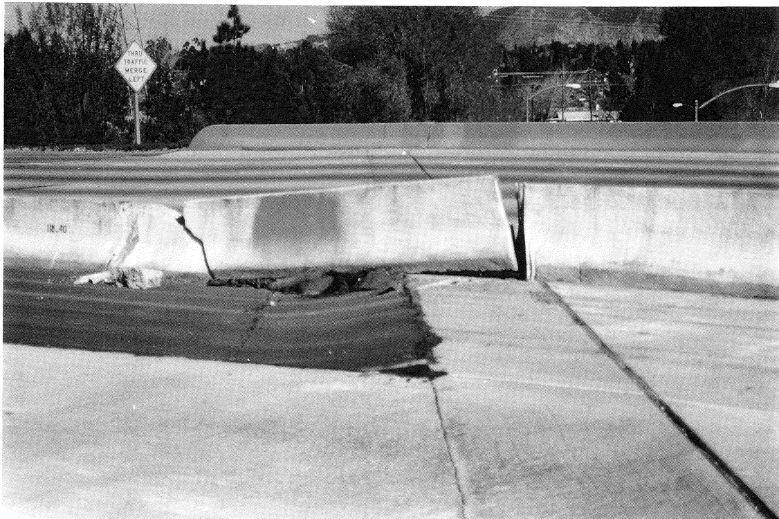
(b) Slumping of Abutment Fills under Roadway Shoulders; Approach Slab in Foreground Successfully Spans Settlement
