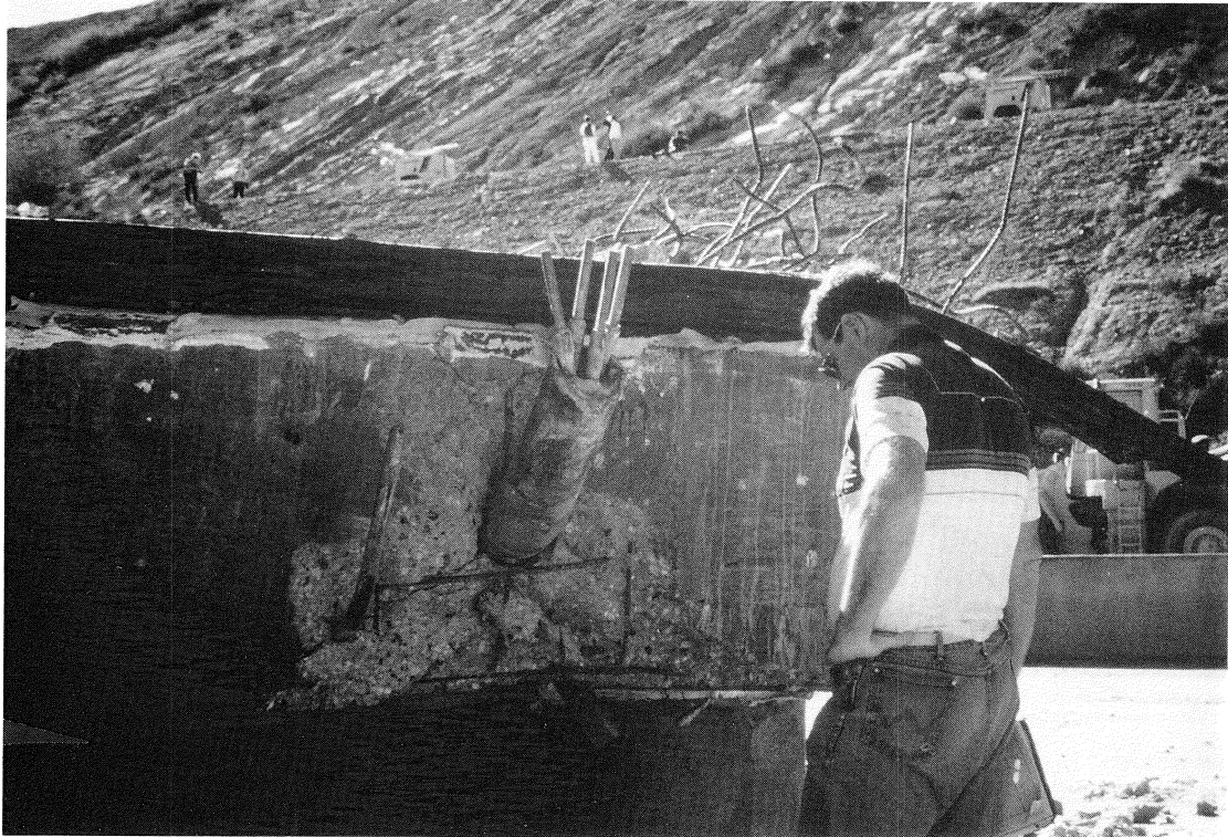
FIGURE 4-10 SR14/I-5 Separation and Overhead (Southbound) - Equalizing Bolt and Restrainers at Hinge in Span 3
