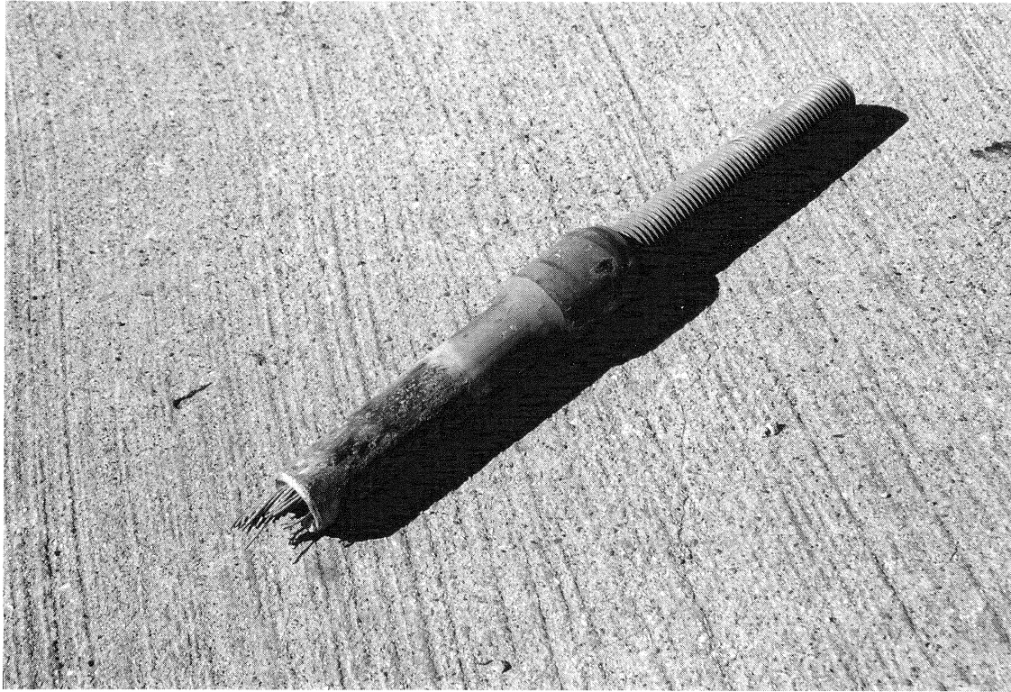
FIGURE 11-1 SR14/I-5 Interchange - Failure of a Type I Hinge Restrainer at the Swaged Fitting
