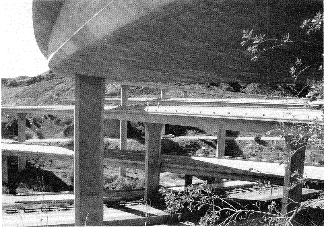
FIGURE 4-1 SR14/I-5 Interchange - General View from Abutment 10 of the South Connector Looking Southwest
