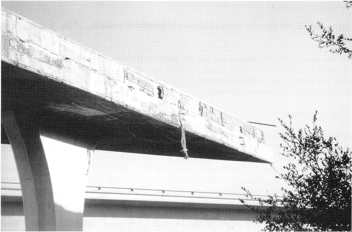
FIGURE 3-5 Gavin Canyon Undercrossing - Hinge Seat and Failed Cable Restrainer
