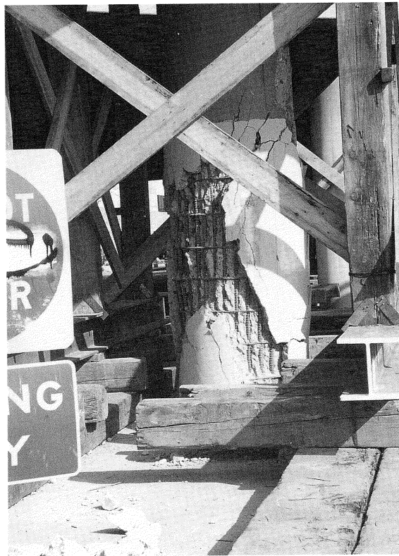
FIGURE 10-7 La Cienega-Venice Undercrossing - Shear Cracking in Column in Bent 8
