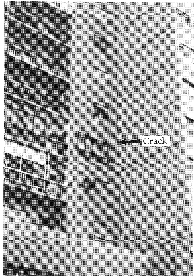
Figure 3-5: Vertical crack in a 36-story shear wall concrete building due to building irregularity.
