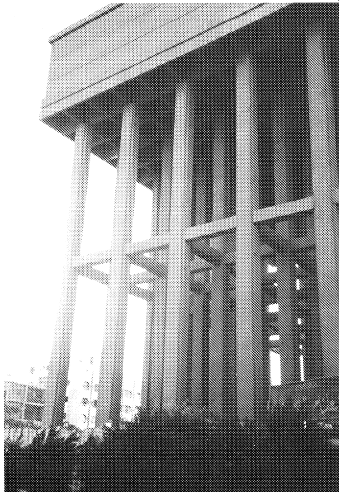
Figure 3-12: The roofing system of this elevated water tank in the City of Giza was damaged during the earthquake.
