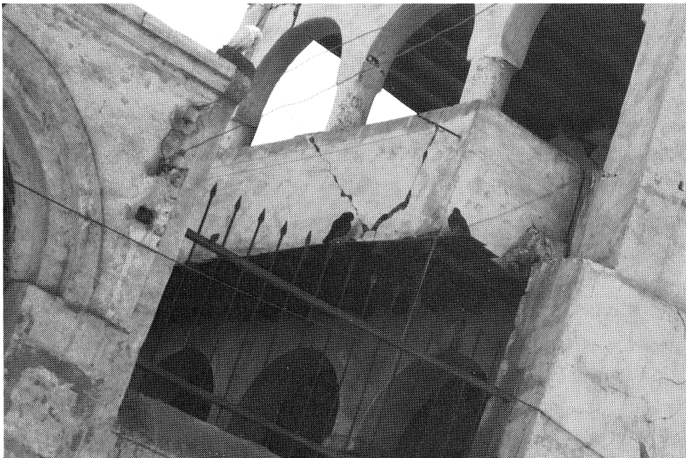
Figure 3-1b: Damage to unreinforced masonry buildings.
