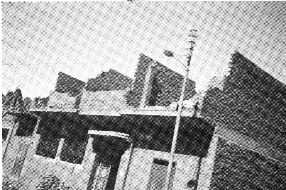
Figure 3-1a: Damage to unreinforced masonry buildings.
