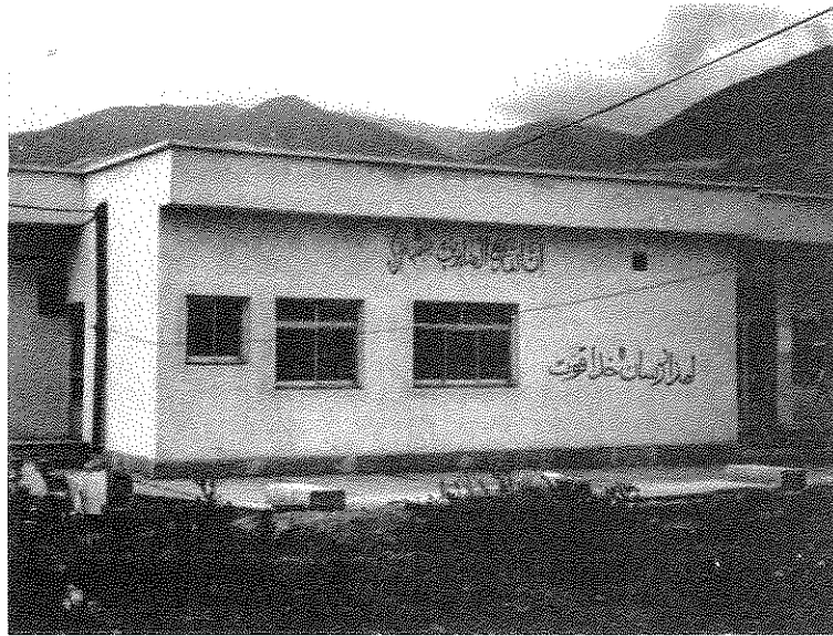
Figure 3-7 Post office building in the area of high ground motion appears to be undamaged
