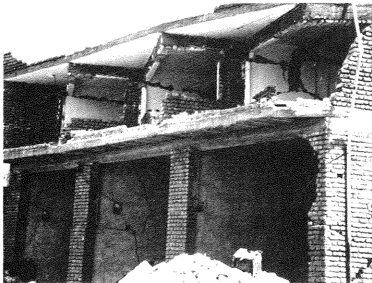
Figure 3-6 Building of Figure 3-5. Presence of reinforced concrete bond beam prevented roof collapse
