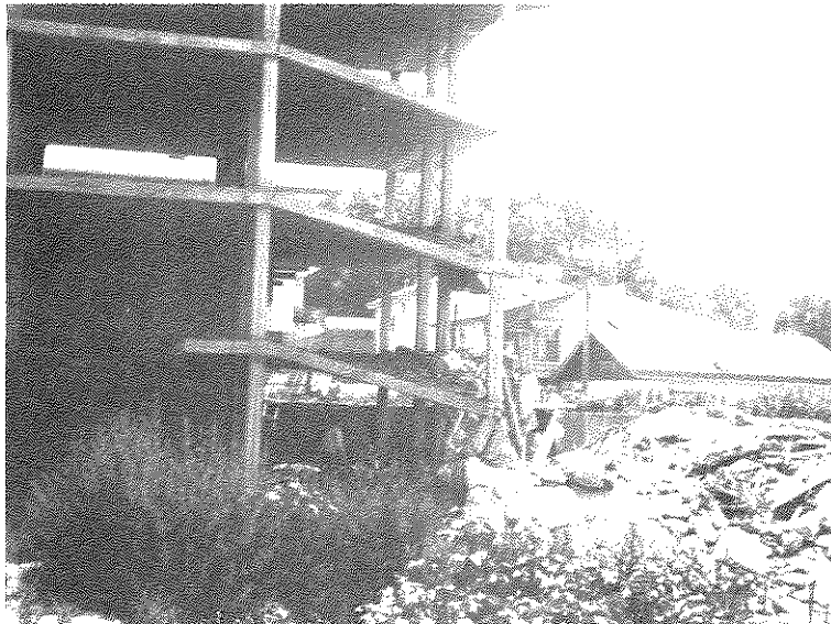
Figure 3-15 Collapse of a mid-rise concrete building and damage to the adjacent building.
