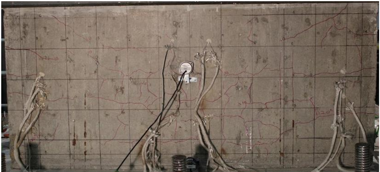
Figure 4-20. Crack pattern on West face of Wall 3 after LC3
