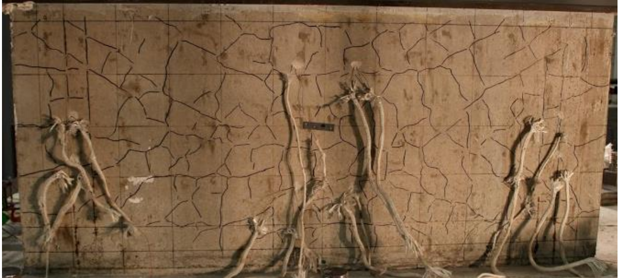
Figure 4-27. Crack pattern on west face of Wall 4 after LC3
