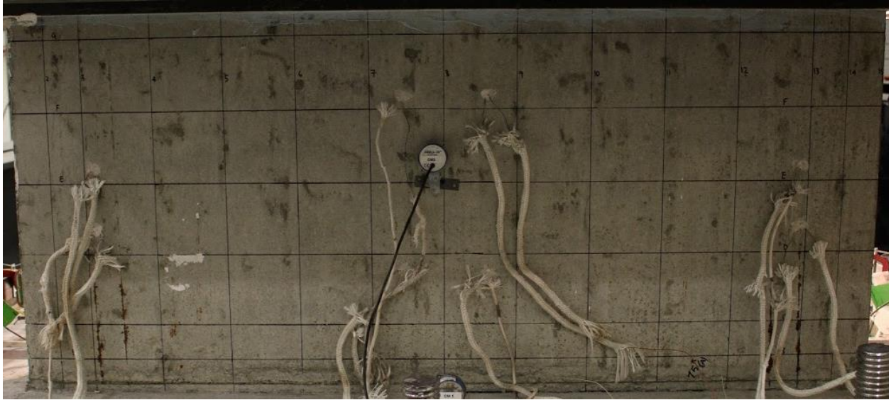
Figure 4-26. Crack pattern on west face of Wall 4 after LC1
