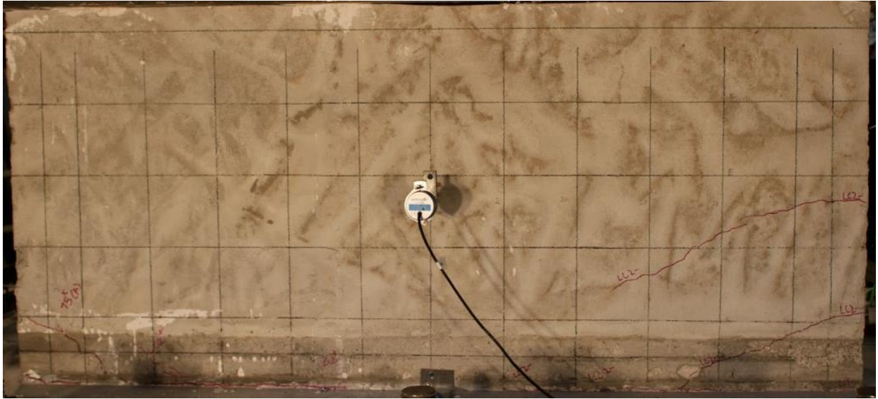
Figure 4-5. Crack pattern on East face of Wall 1 after LC2
