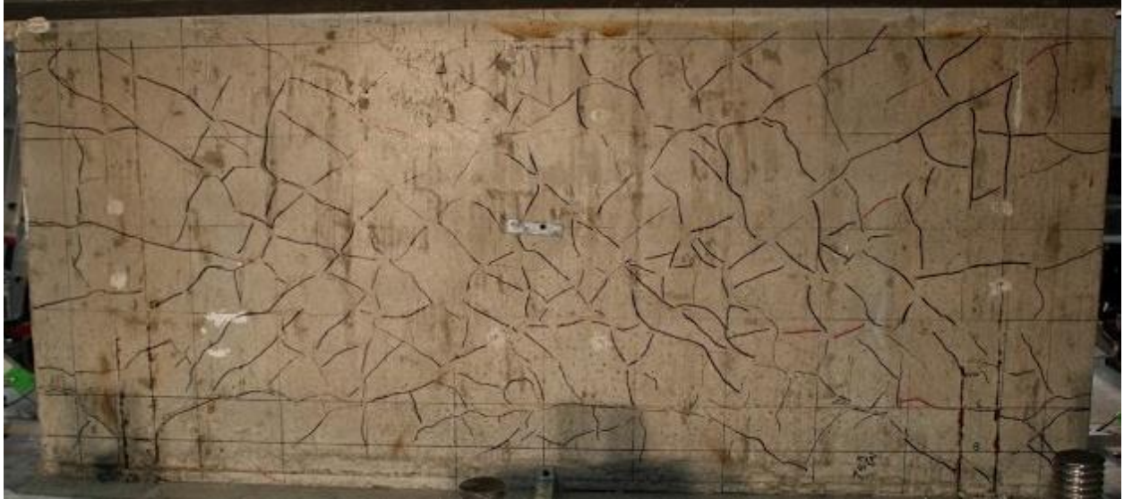
Figure 4-28. Crack pattern on west face of Wall 4 after LC15
