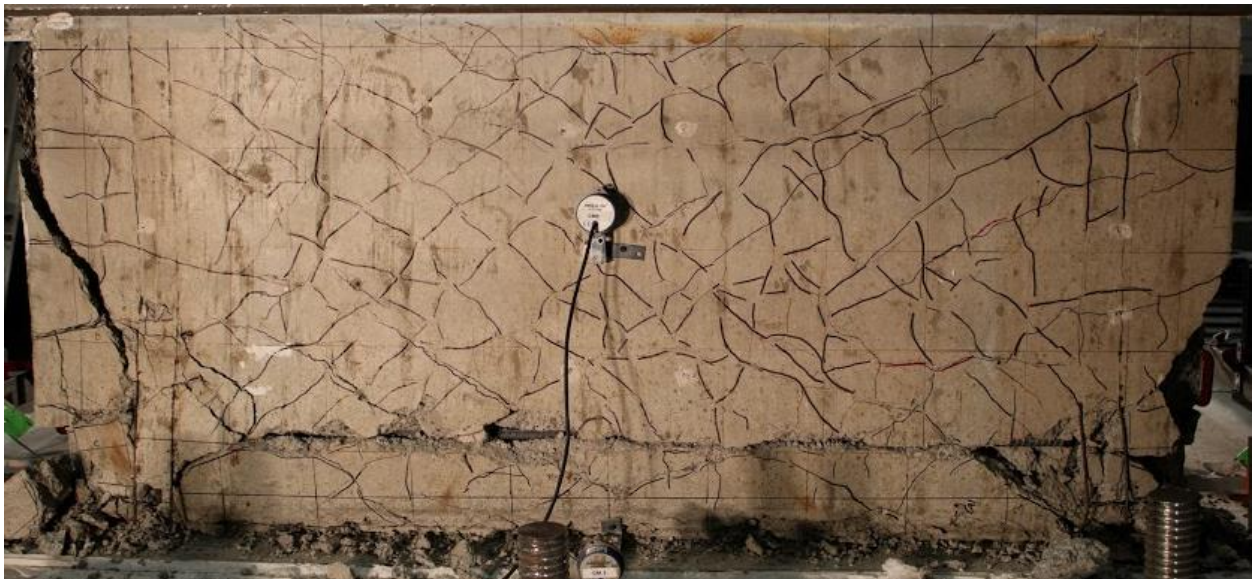
Figure 4-29. Damage to Wall 4 at the end of testing
