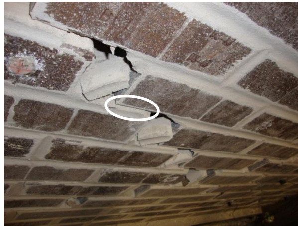
Figure 8-67. Out-of-plane gap in the joints at the end of the test
