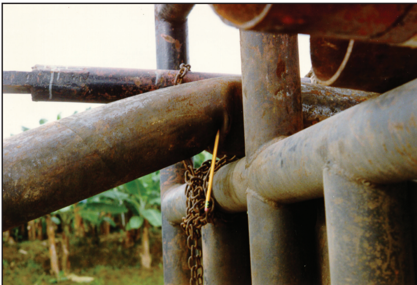
■ Figure 4.1 Pencil in Tear at Wrinkle in RECOPE Pipeline (Limon, Costa Rica, 1991)
