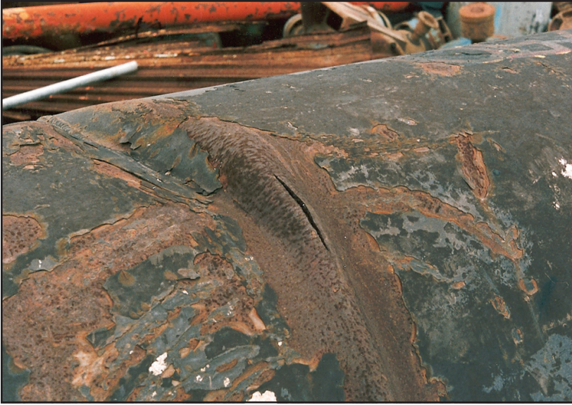
■ Figure 4.2 Tear at Wrinkle in Ciudad Nezahualcoyotl Pipeline (Mexico City, 1985)
