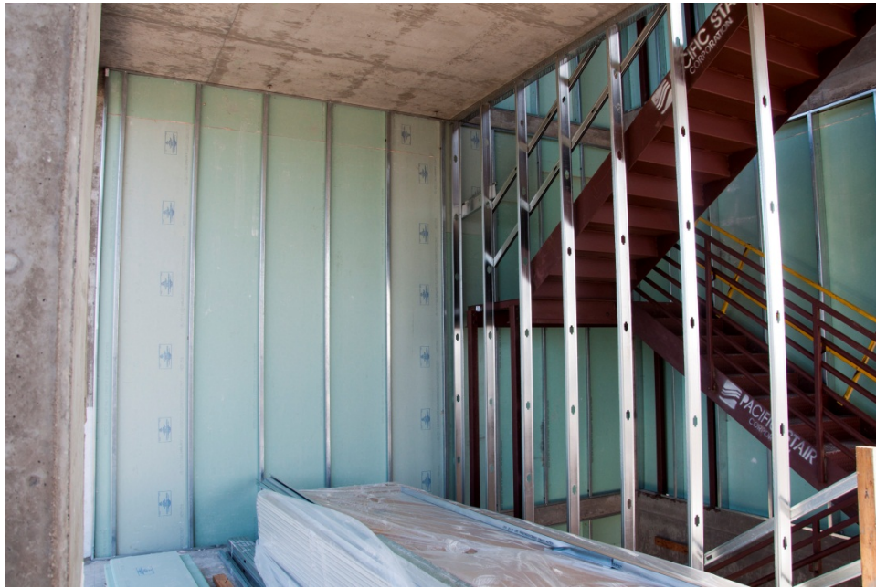
Figure 8-1 Example usage of light-gauge steel studding and gypsum board system during construction.
