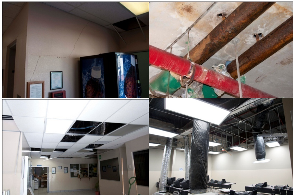
Figure 1-1 Examples of nonstructural failures from the 2010 Baja California Earthquake ( M_w=7.2 ). Partition wall and pipe failures at El Centro Regional Medical Center (upper) and ceiling fallout and HVAC system failure at Universidad Autónoma de Baja California in Mexicali, BC (lower).
