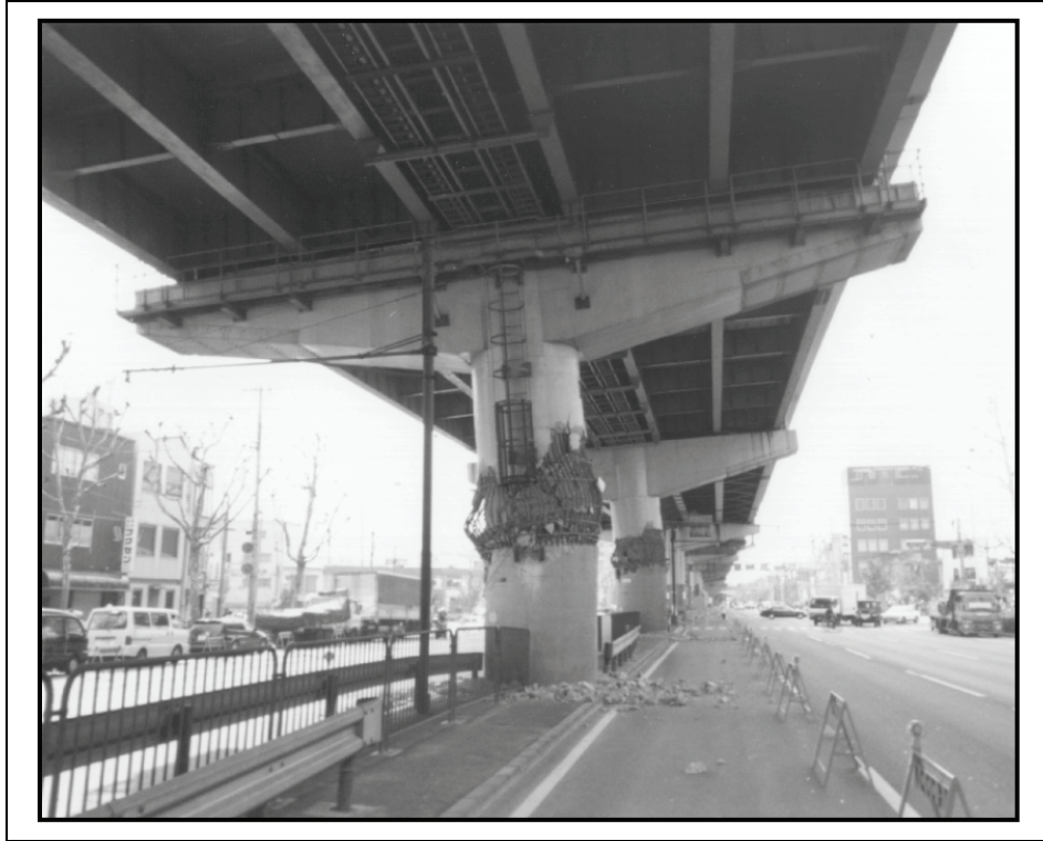
Figure 5-29. Severe Damage: Mid-height Flexural Damage (PEQIT)
