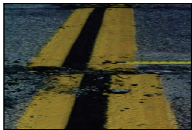
Figure 5-37: Minor Damage: Transverse Movement Along the Centerline (COHMR)
