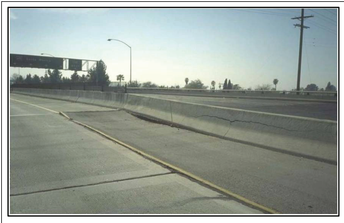
Figure 5-7. Moderate Damage: Approach Slab Settlement (Sardo, A. G., et al., 2006). Note the cracking of the concrete barrier as well.
