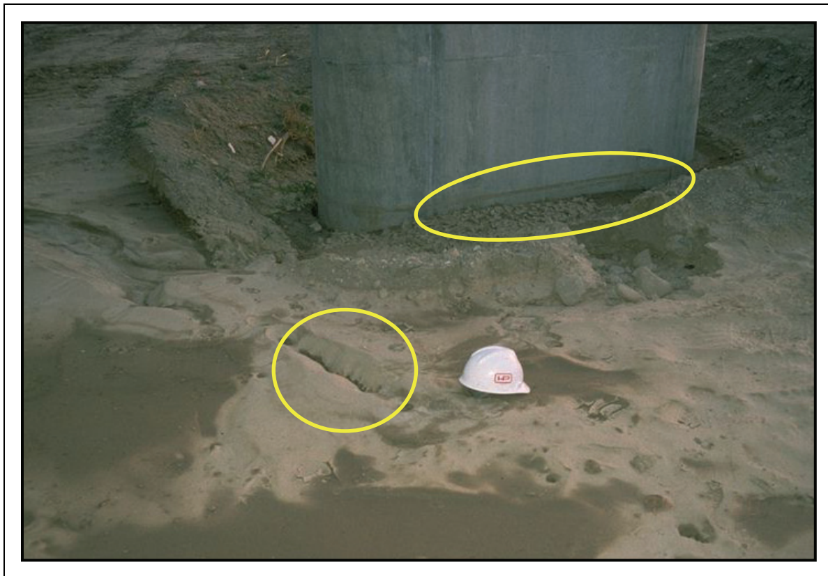
Figure 5-10. Evidence of Liquefaction near a Pier (NISEE)
