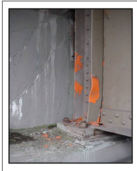
Figure 5-15. Minor Damage: Web Stiffener Damage. Note that the paint has flaked off recently. (MCEER)
