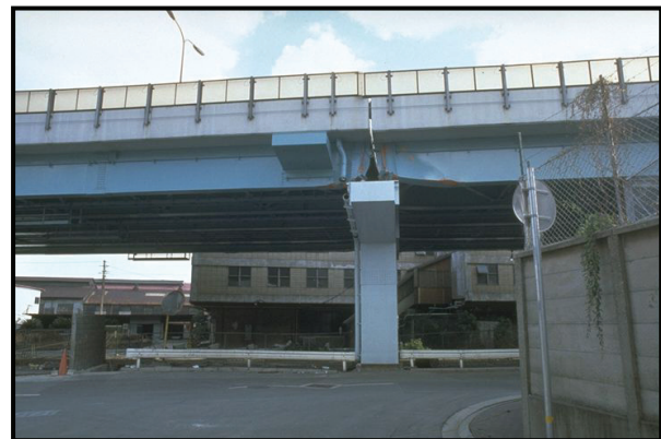
Figure 5-19. Severe Damage: Steel Girder Buckling (MCEER)
