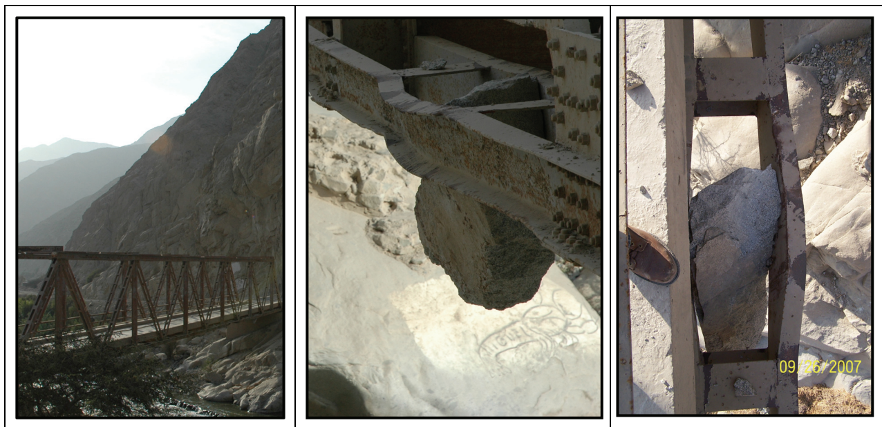
Figure 2-1. Damage from Rockfall in Peru. (O'Connor)
