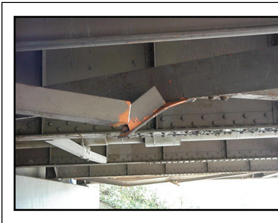
Figure 5-18. Moderate Damage: Fracture of Lower Lateral Bracing (MCEER)
