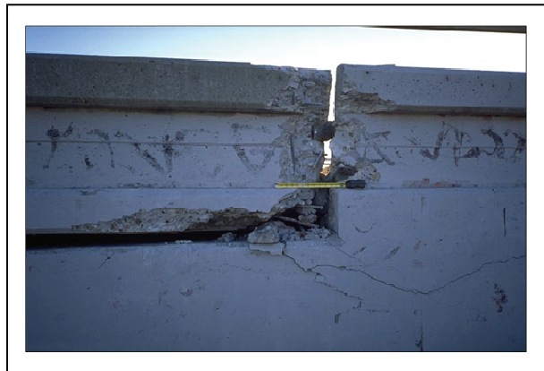
Figure 5-4. Evidence of Longitudinal Pounding (NISEE)
