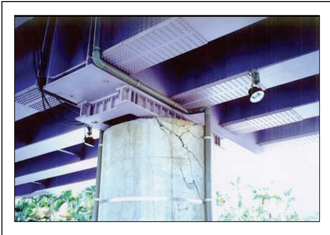
Figure 5-27. Moderate Damage: Compression Failure at Top of Concrete Column (INDOT)
