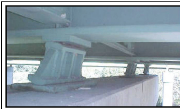
Figure 5-39. No Damage: Tilted Rocker Bearings, Movement Due to Thermal Loads (INDOT)
