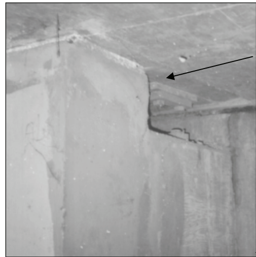
Figure 5-44. Severe Damage: Missing Abutment Bearing after Northridge (PEQIT)
