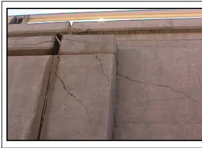
Figure 5-45. Minor Damage: Shear Cracking at the Abutment Wing-wall (KTC)
