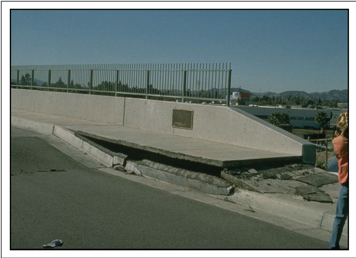
Figure 5-11. Settlement at the Bridge Approach, Likely Caused by Soil Settlement around the Abutment (Northridge EQ) (NISEE)
