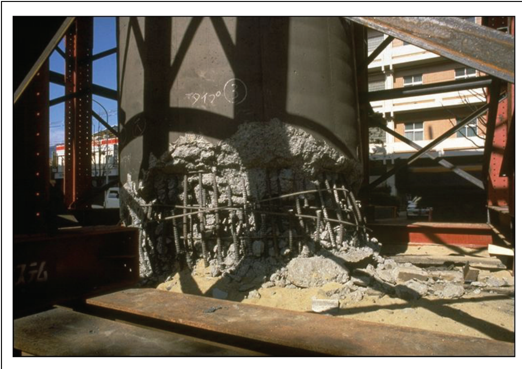
Figure 5-34. Severe Damage: Weld Failure of Column Longitudinal Reinforcement (MCEER)
