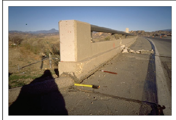
Figure 5-3. Settlement at Approach: Spalling (NISEE)
