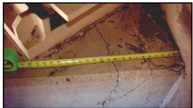
Figure 5-40. Minor Damage – Cracks Induced by Steel Bearing (CPHMR)
