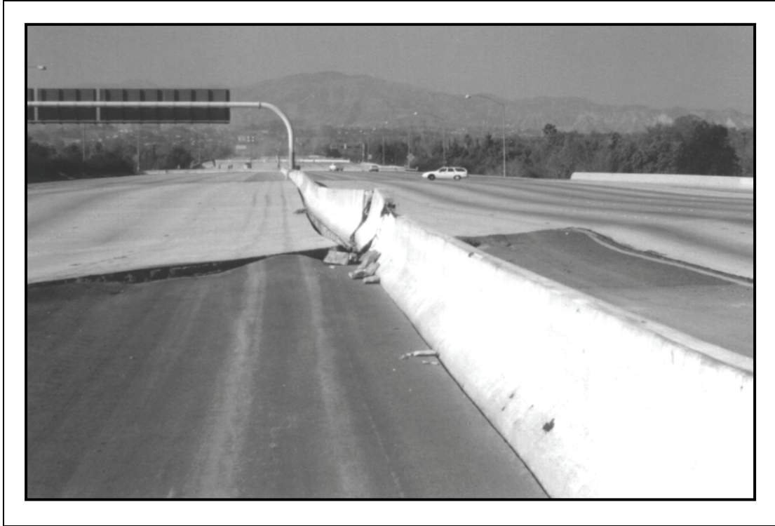
Figure 5-8. Approach Damage Considered Moderate to Major (Northridge Earthquake) (PEQIT)
