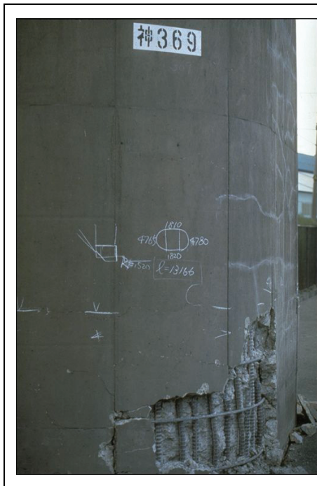
Figure 5-30. Moderate to Severe Damage: Spalled Column; Buckling of Primary Reinforcement (MCEER)
