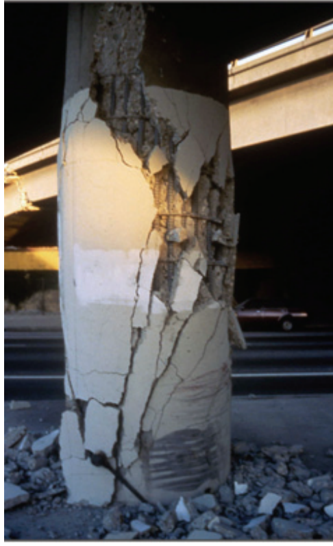
Figure 5-53. Earthquake Damage to Reinforced Concrete Bridge Column (Aboutaha)
