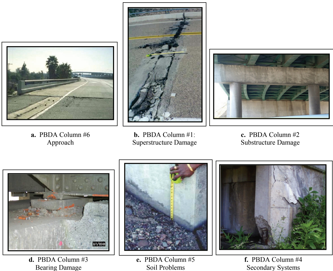
Figure 5-1. Photographic examples of bridge damage for inclusion in a Preliminary Bridge Damage Assessment (PBDA) – (NISEE)
