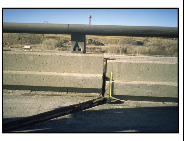
Figure 5-21. Minor to Moderate Damage: Vertical and Horizontal Movement at Joint (NISEE)
