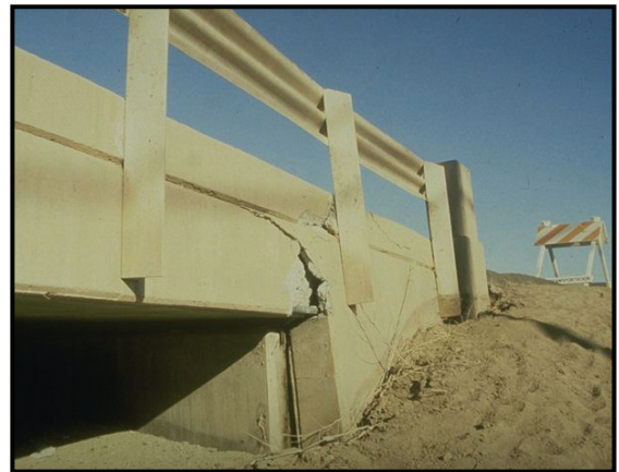
Figure 5-46. Moderate Damage: Abutment Slumping and Rotation Failure (NISEE)
