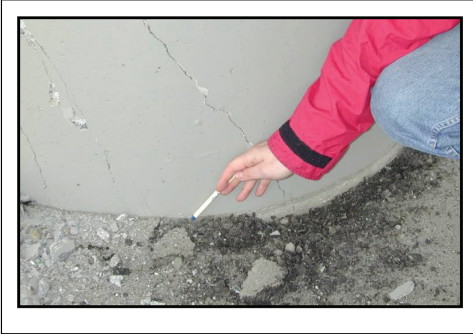
Figure 5-25. Ground Movement Indicating Possible Foundation Problem (MCEER)
