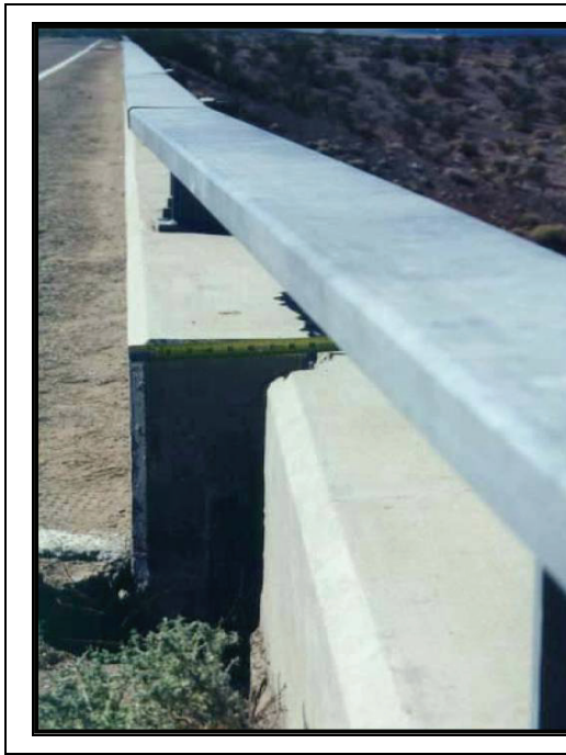
Figure 5-51. Moderate Damage: Transverse Movement of the Abutment Wing-wall (CPHMR)
