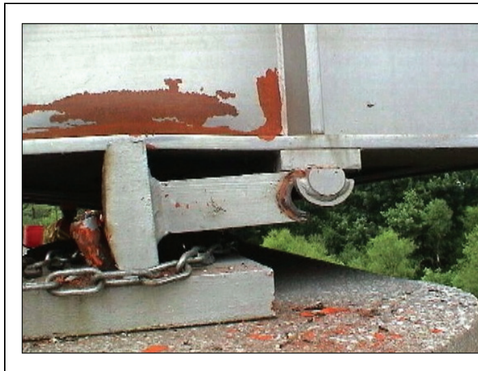
Figure 5-43. Severe Damage: Rocker Bearing Failure (MO)
