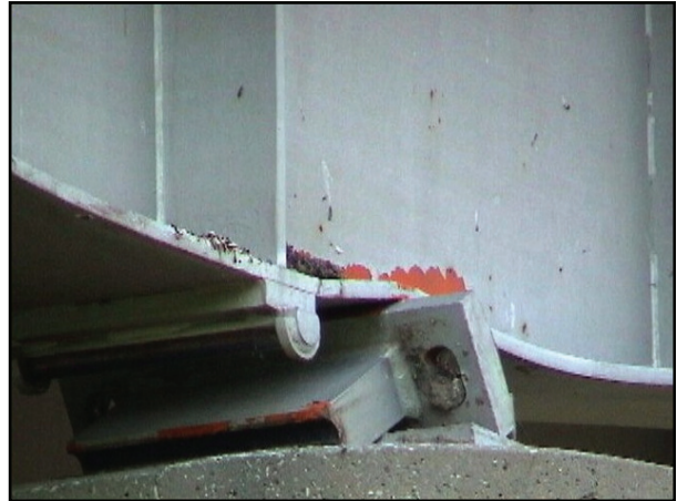
Figure 5-42. Severe Damage: Toppled Rocker Bearing (MO)
