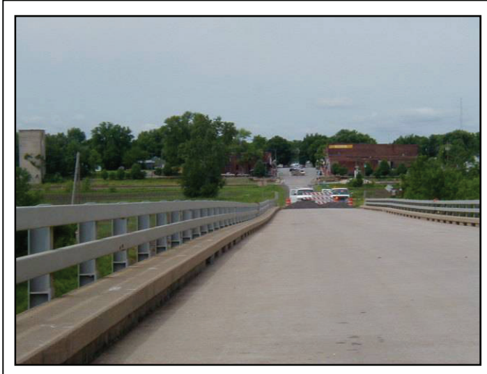
Figure 5-48. Moderate Damage: Bowing of Parapet and Railing (MO)
