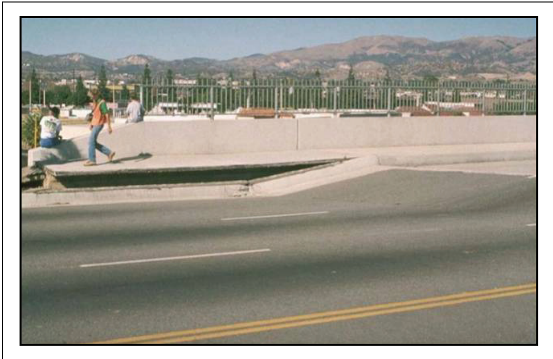
Figure 5-9. Settlement of Bridge Approach, Considered Major Damage (KTC)
