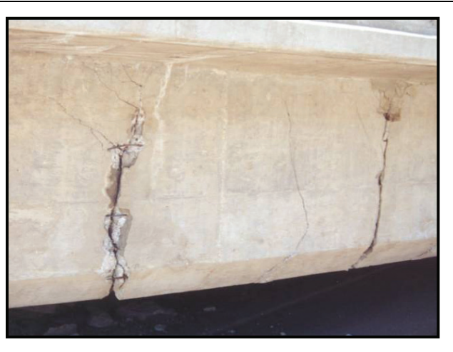
Figure 5-13. Moderate Damage: Flexural Cracking of Concrete Girder (KTC)
