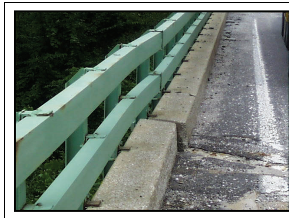
Figure 5-49. Misalignment of Curb Line and Bowing of Railing. Notice that the white edge line is slightly shifted at the joint. (MO)
