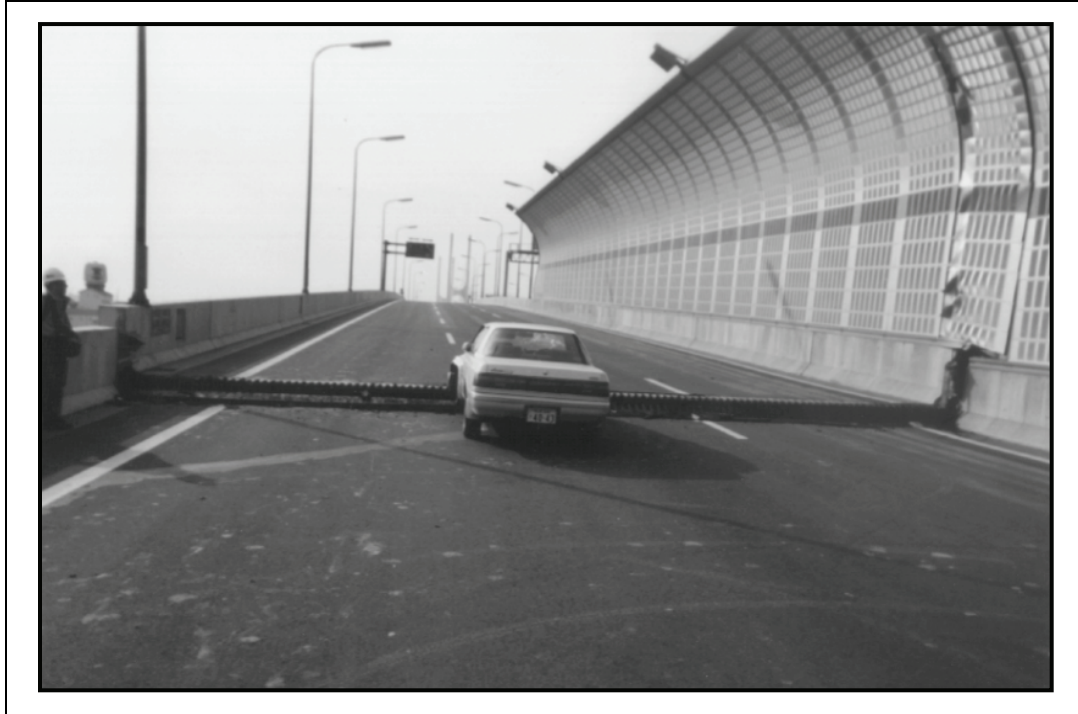
Figure 5-38: Moderate Damage: Differential Settlement and Expansion Joint Damage (PEQIT)
