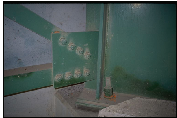
Figure 5-17. Minor Damage: Damage to Anchor Bolts (MCEER)
