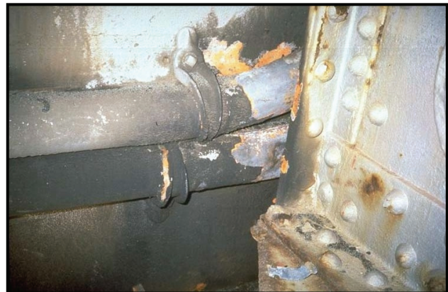
Figure 5-50. Movement of Trusses at Pier 23 of the San Francisco Oakland Bay Bridge during the Loma Prieta Earthquake. The shoe (at the right) hit two pipes that carried electric wires and dented them. These dents indicated that there was at least 3 to 4 inches of movement. (NISEE)
