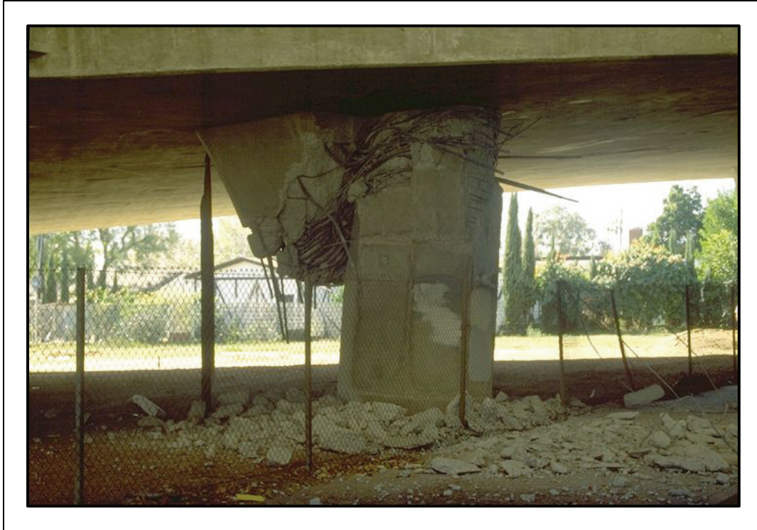
Figure 5-35. Severe Damage: Shear Failure (1971 San Fernando Earthquake) (MCEER)
