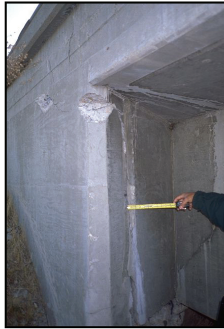
Figure 5-52. Minor Damage: Wing-wall and End-wall (CPHMR)
