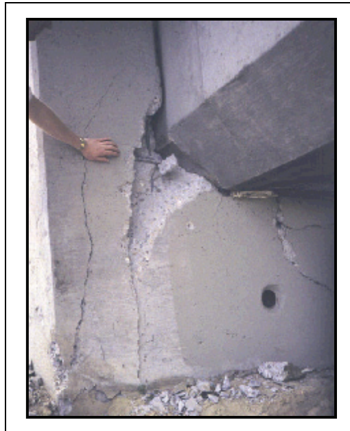
Figure 5-47. Moderate Damage: Spalling and Cracking of Abutment, Movement at Ground Level (MO) Note that the rebar is not rusting, an indication that damage is recent.
