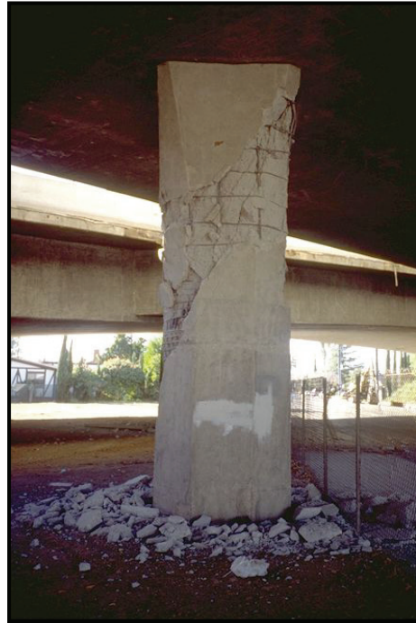
Figure 5-33. Severe Damage: Brittle Shear Failure (NISEE)
