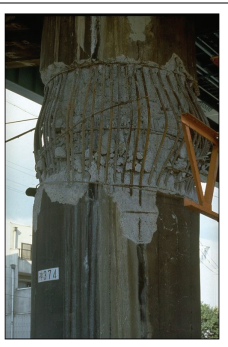
Figure 5-31. Severe Damage: Confinement Failure (MCEER)
