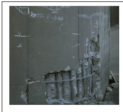
Figure 5-5. Spalling and Splice Failures at Column Base (NISEE)
