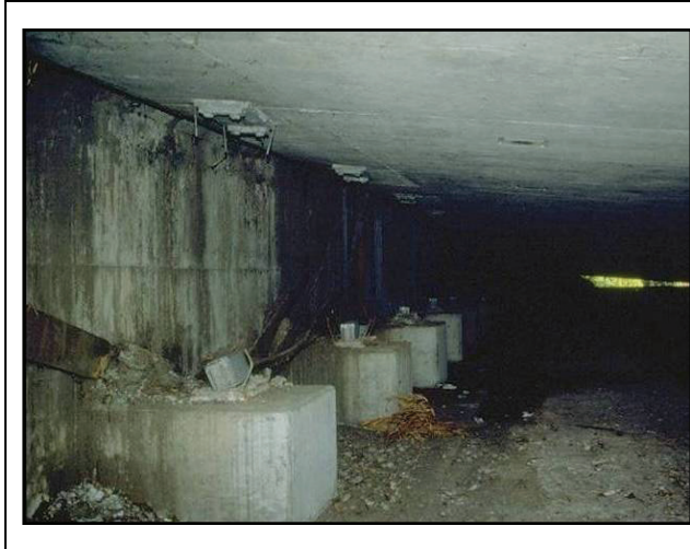
Figure 5-41. Moderate Damage: Abutment Rocker Bearings. (MCEE)
