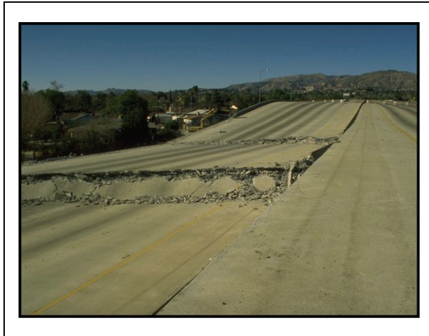
Figure 5-22. Severe Damage: Deck Collapse (KTC)
