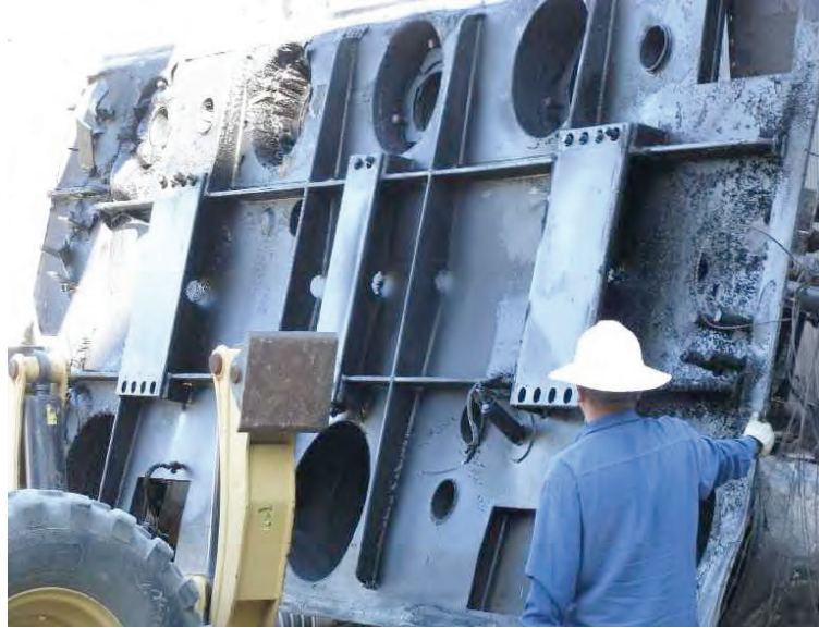
Figure 3-4 Underside of 230kV Transformer Cover showing Stiffening Members (courtesy of Schiff, 2011)
