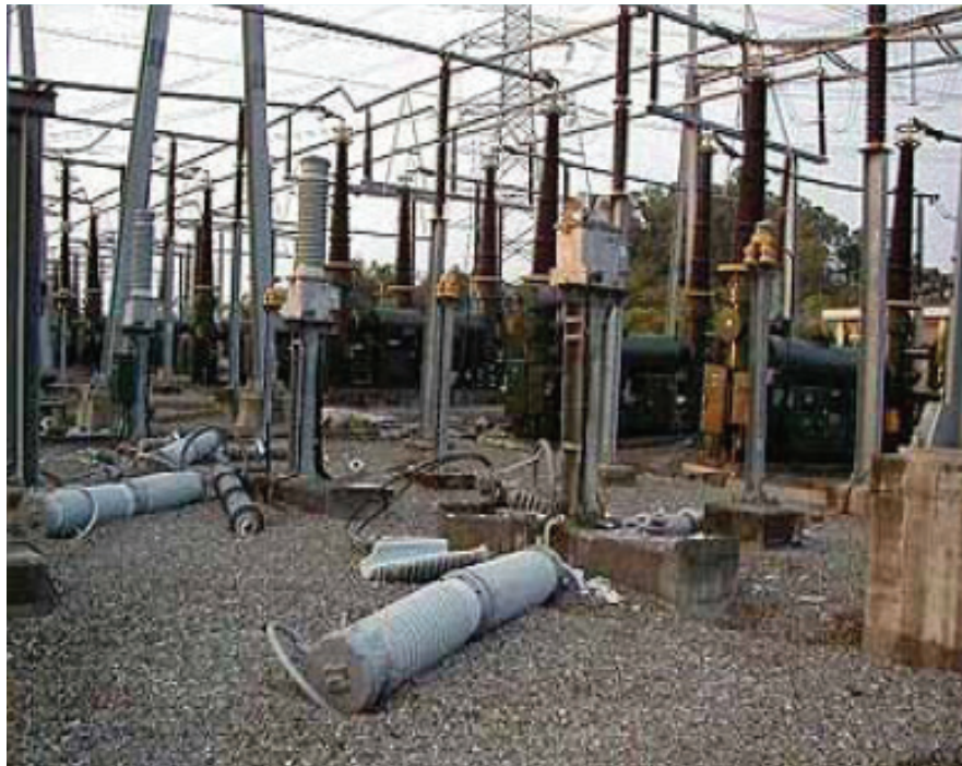
Figure 1-7 Bushing Failure, Taiwan 1999 (Wang, 2008)
