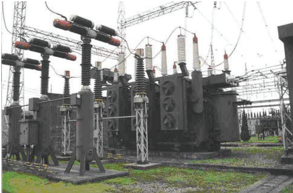
Figure 1-1 Typical Electrical Substation (Ersoy et al., 2008)
