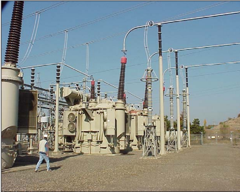
Workshop on Improving Seismic Response of Substation Equipment – 10/24/2008
