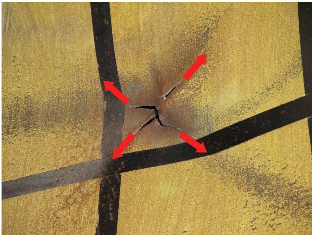
(b) Detail of Panel Tear
