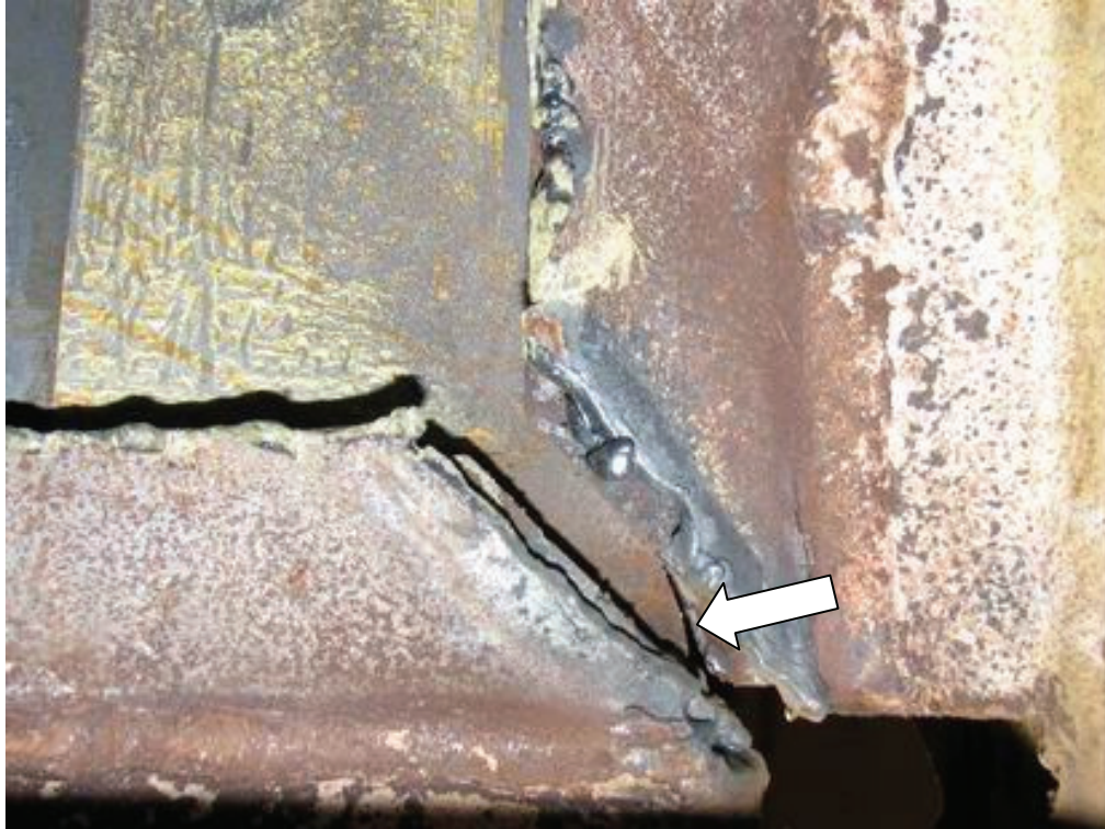
(a) Onset of the Panel Tear
