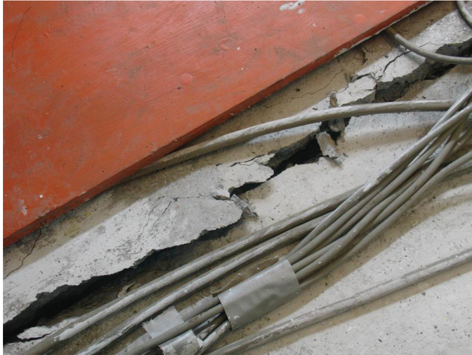
(a) Crack along the Intermediate HBE
