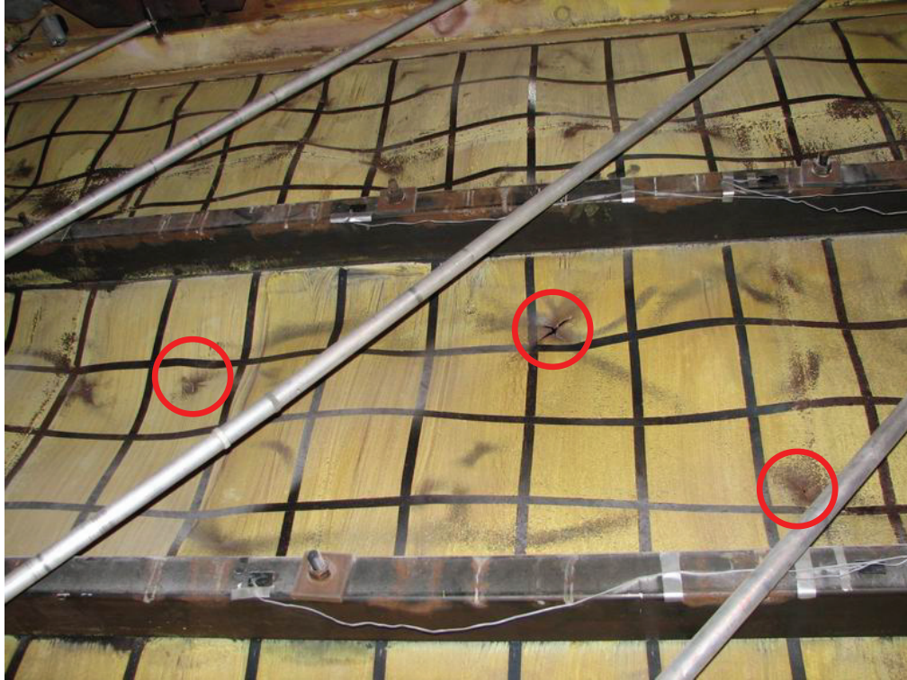
(a) Overall View of Panel Tear
