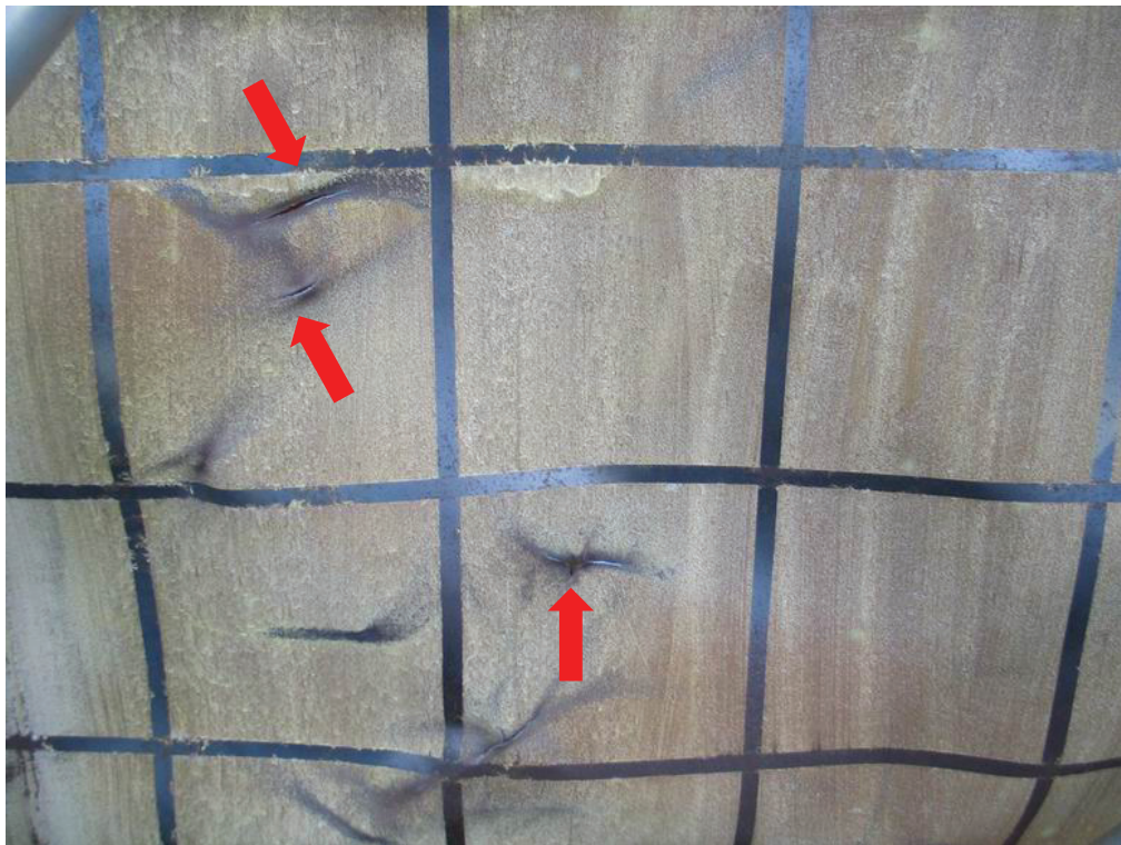
FIGURE 4-16 Initiation of the Panel Tear
