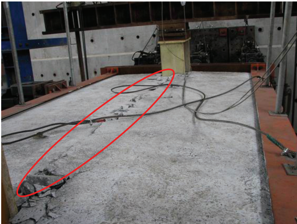
FIGURE 4-60 Crack in the Top Concrete Slab
