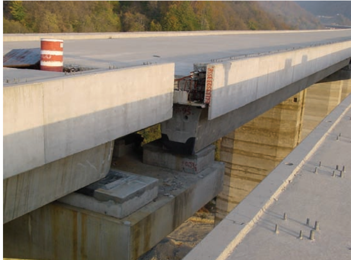
Figure 2-7. Damage Sustained by the Bolu Viaduct during Duzce Earthquake 1999
