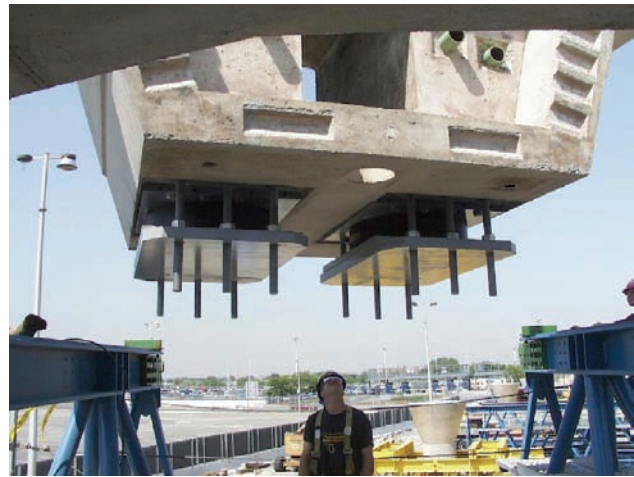
Figure 2-3. Lead-rubber Isolators being Installed in the JFK Airport Light Rail Viaduct, New York
