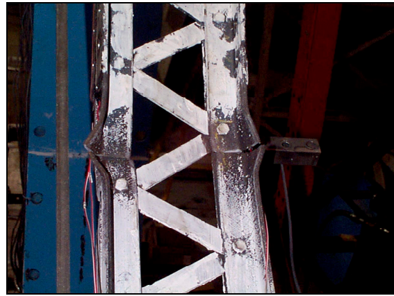
Figure 22. Fracture of Ay8-120
