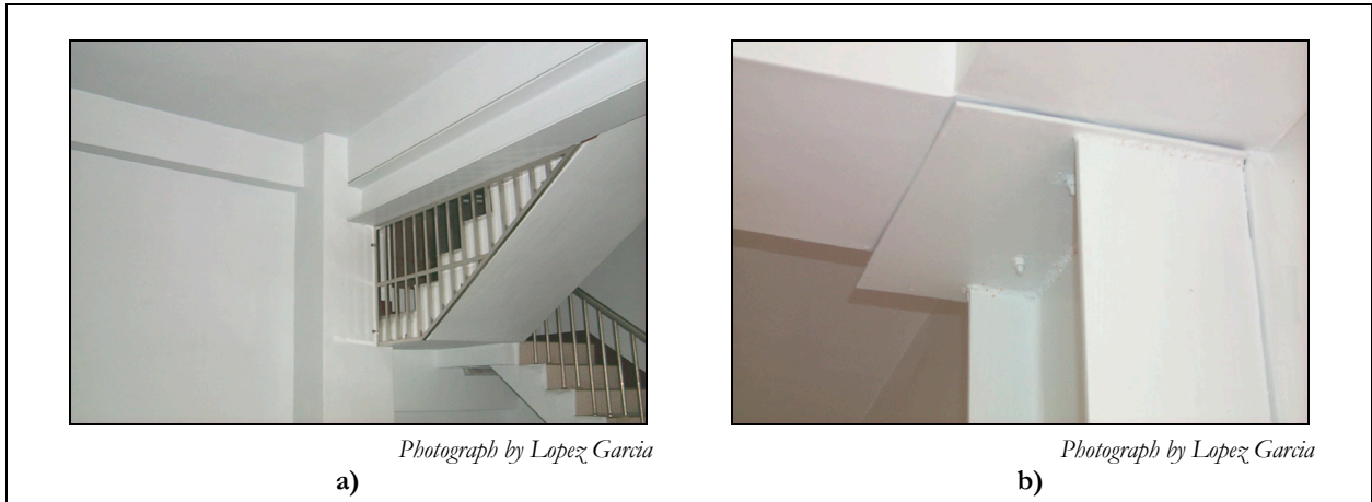
Figure 3. Non-engineered retrofit of residential buildings: (a) RC beam strengthened by a steel beam; (b) eccentric RC beam-column joint supported by a steel column
