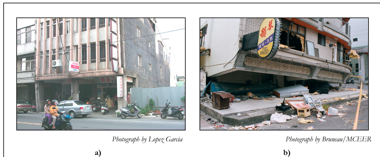
Figure 1. Typical residential building in Taiwan: (a) pedestrian corridor and open front; (b) soft story damage
