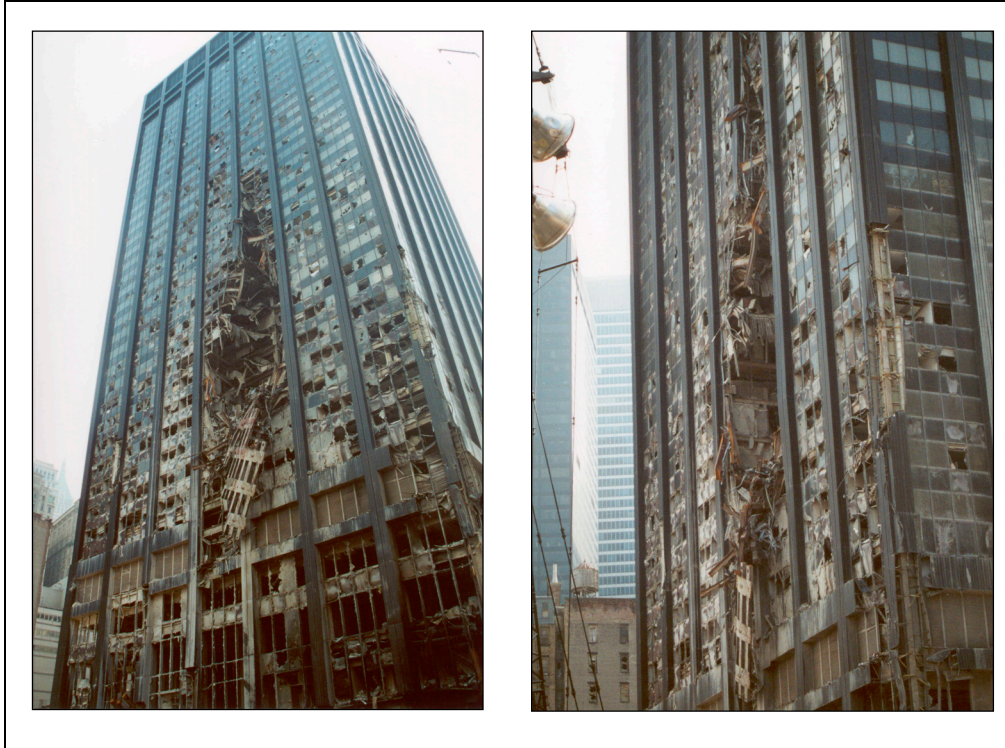
Figure 1. Building damage to northern façade and column on line D
