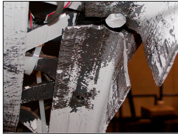
Figure 24. Fracture of Ay16-120
