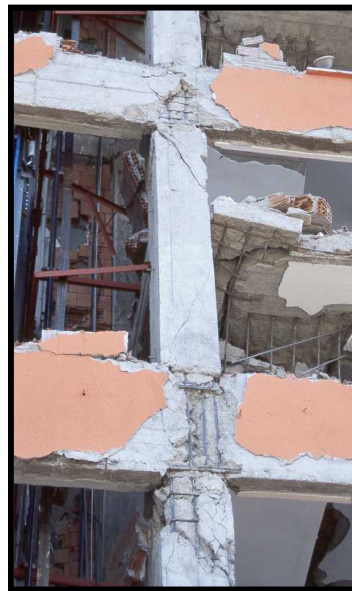
Figure 1b: Damage after the 1999 Turkey earthquake (NISEE).
