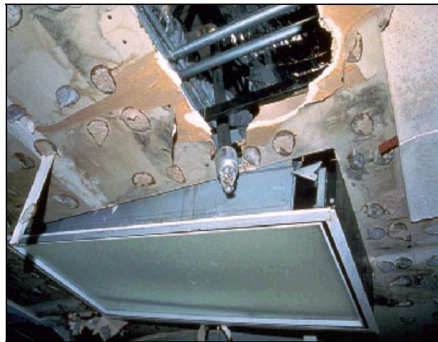
Figure 2 – Damaged ceiling, sprinkler pipe, and lighting fixture; Northridge Earthquake, Jan. 1994.
