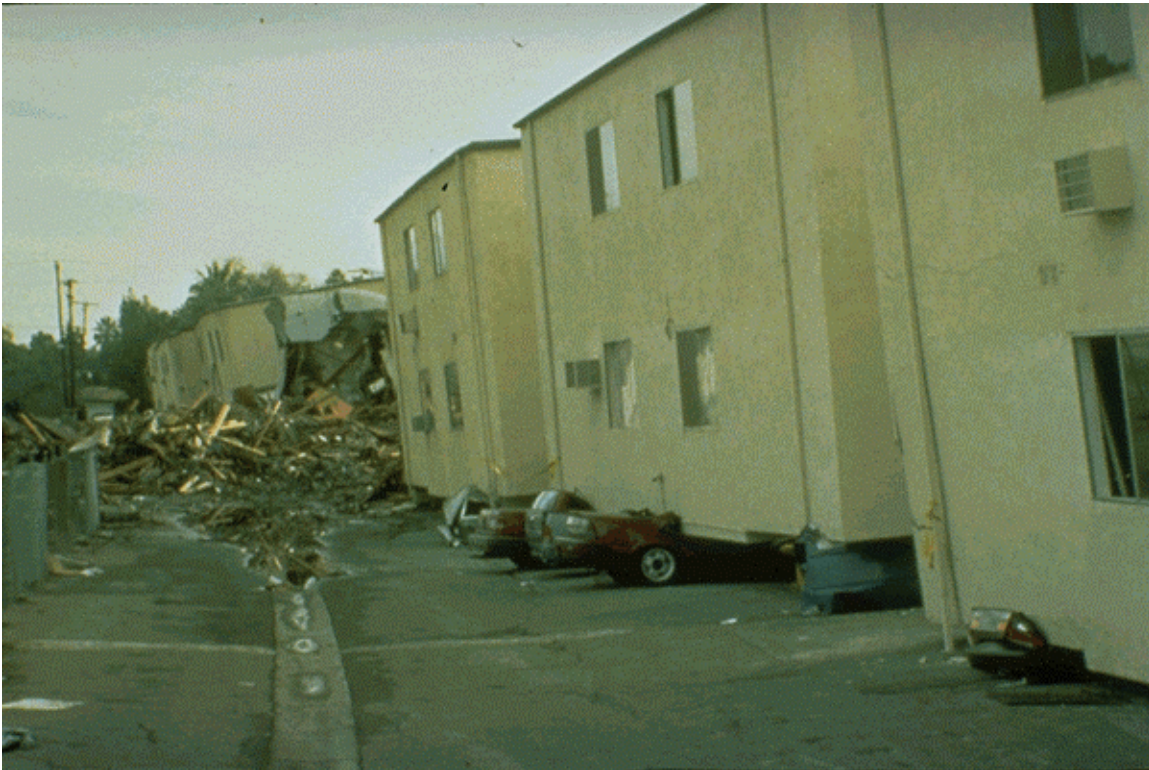
Figure 1: Collapsed first story of California apartment
