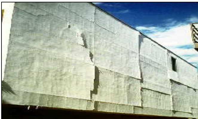
Figure 9 – Stucco damage on the façade of the South Library at Cal State University; Northridge, Jan 1994.
