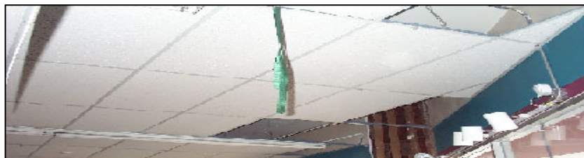
Figure 7 - Ceiling damage to department store in Olympia, WA; Nisqually Earthquake Feb. 2001.
