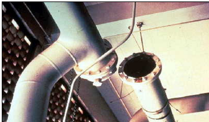
Figure 5 – Seismic damage to piping joint at the original Olive View Hospital, San Fernando Earthquake, Feb. 1971.
