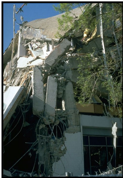
Figure 1a: Damage after the 1994 Northridge earthquake (NISEE).
