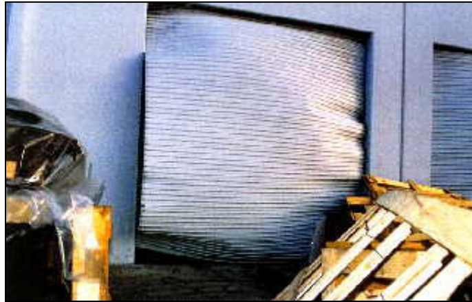
Figure 4 - Severe damage to roll - up door in a tilt-up warehouse; Northridge earthquake, Jan. 1994.
