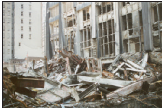
d. Damage to the northern façade at the entry level
