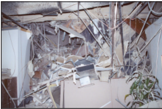
a. Complete destruction of one zone of the building
