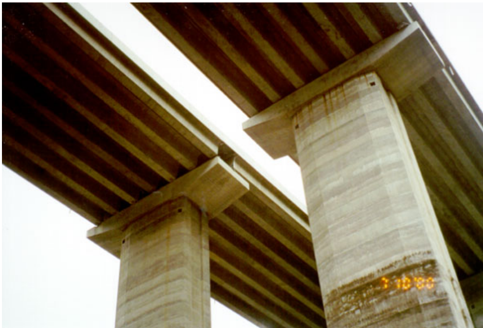
Figure 2-10 Close-up View of Girders on Pier Tops Showing Significant Permanent Offset of Girders
