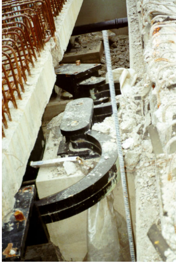
Figure 2-15 View of Energy Dissipating Devices at Expansion Joint Showing Failure of Connections of the Energy Dissipating Device to Deck
