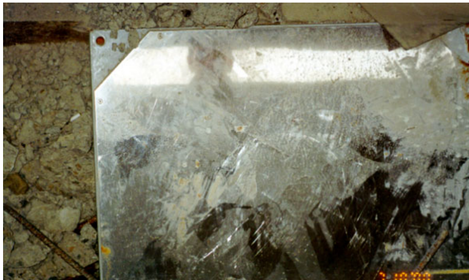
Figure 2-14 Typical Trace on Displaced/Ejected Bearing Plates
