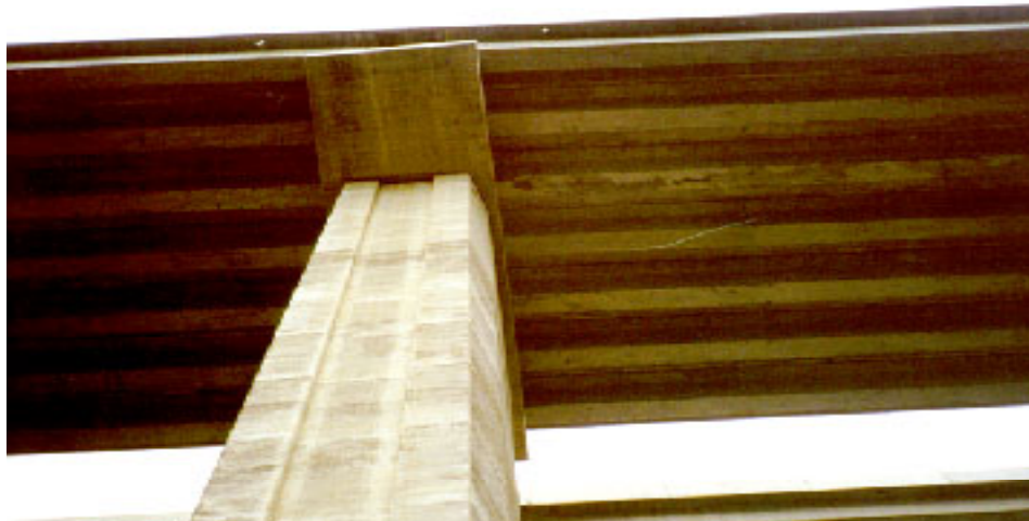
Figure 2-16 Rotation of Pier 45 about Vertical Axis
