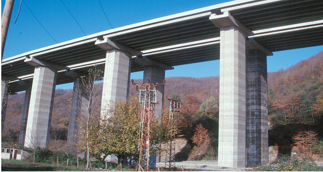
Figure 2-9 Girders Off-Set from their Supports
