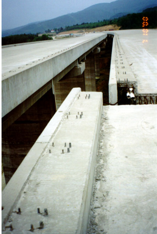
Figure 2-11 Permanent Displacements as Seen at Expansion Joints
