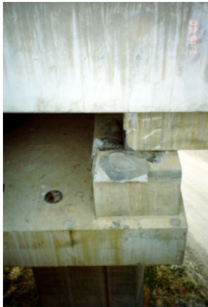
Figure 2-12 Damage and Permanent Displacement at Sliding Bearings
