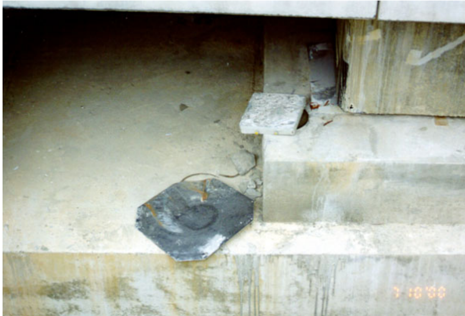
Figure 2-13 Close-up View of Failed Sliding Bearings (Note that Stainless Steel Plate was Ejected from Bearing)
